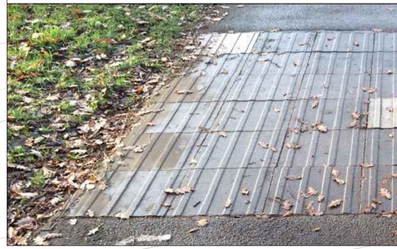
LADDER/TRAMLINE TACTILE PAVING
