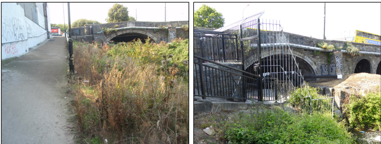
Figure 12: Existing Views from Tow Path on Approach to Binns Bridge & 2 nd Lock
