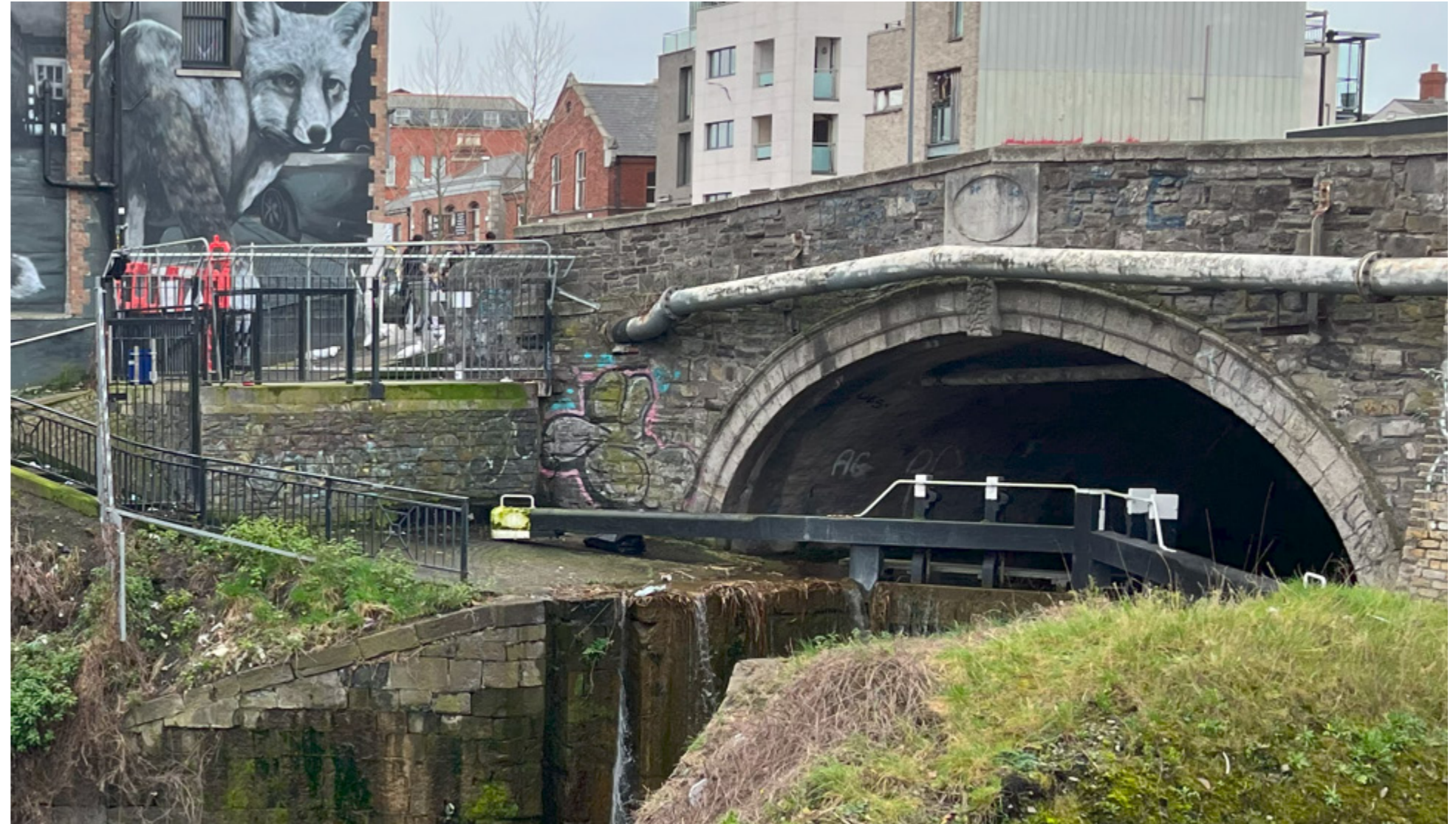
Fig 5. Graffiti on face of bridge stone work to be removed
