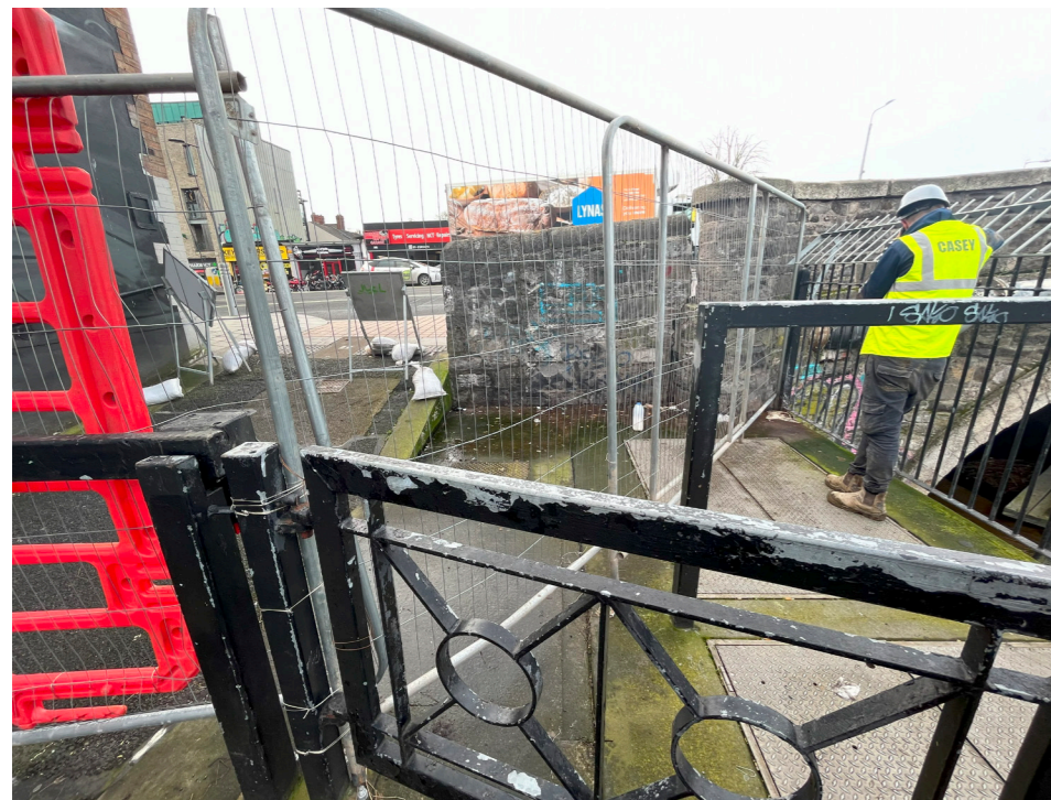
Fig 20. Upper surface of Gas District Regulator installation.
