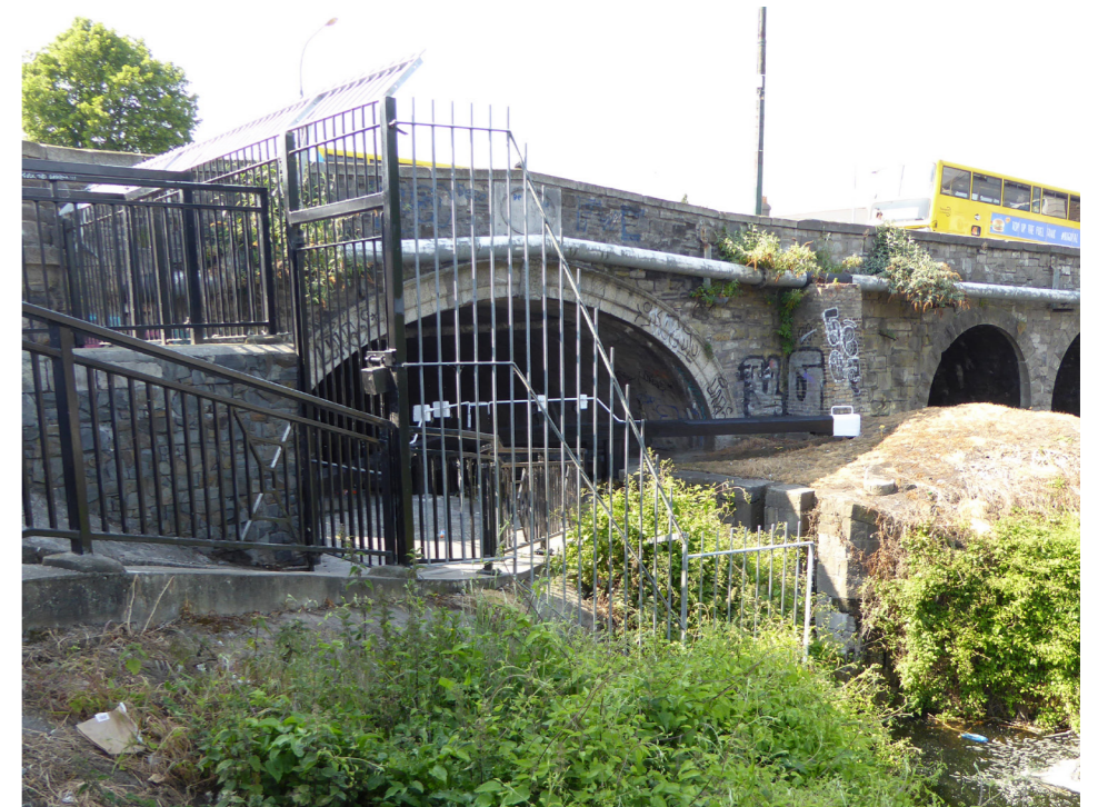
Fig 26. Extensive anti-entry railings create inhospitable atmosphere.
