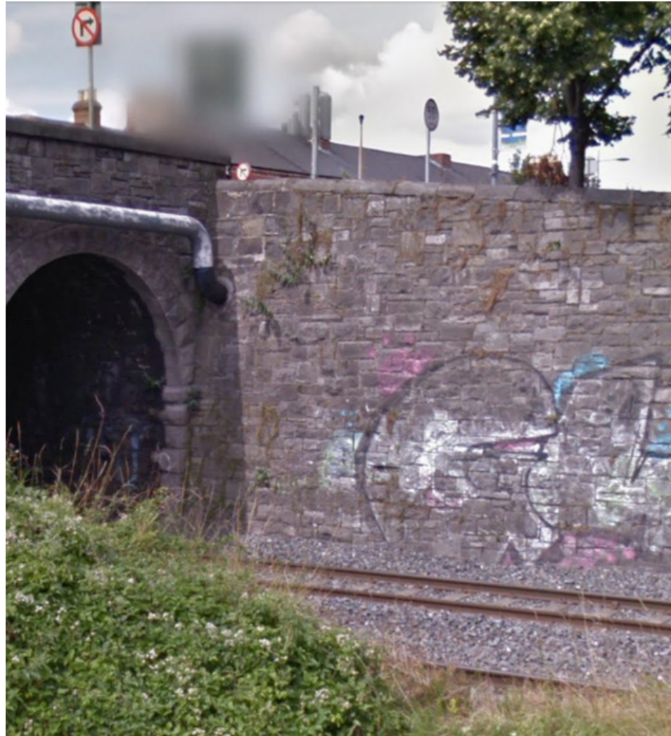
Fig 36. Materiality reference: Masonry calp retaining wall abutting bridge over railway on opposite bank to proposed cycleway.
