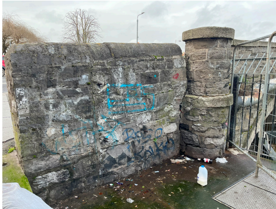
Fig 17. Remnant section of boundary wall to be altered to increase access width.
