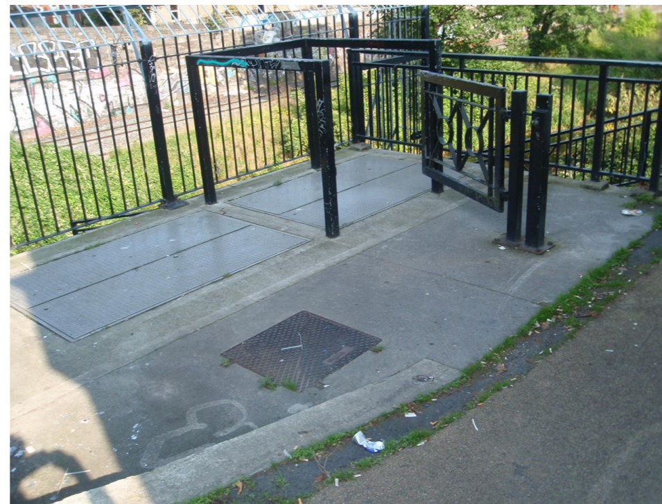
Fig 21. Upper surface of Gas District Regulator installation with railing enclosure.
