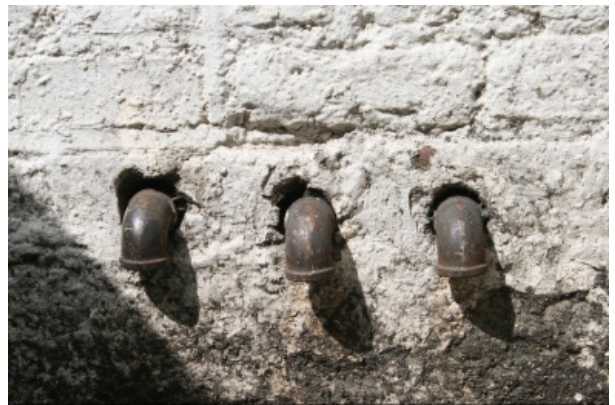
Feature 2: Three metal pipes on Duke Lane (rear of 15-20 Grafton Street)
