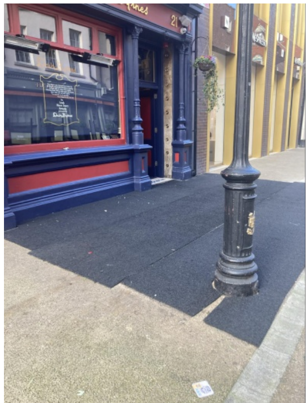
Feature Number: 22 - Left: Original survey photo in 2019. Right: Keg hole now covered outside Davy Byrnes, 18 Duke Street
