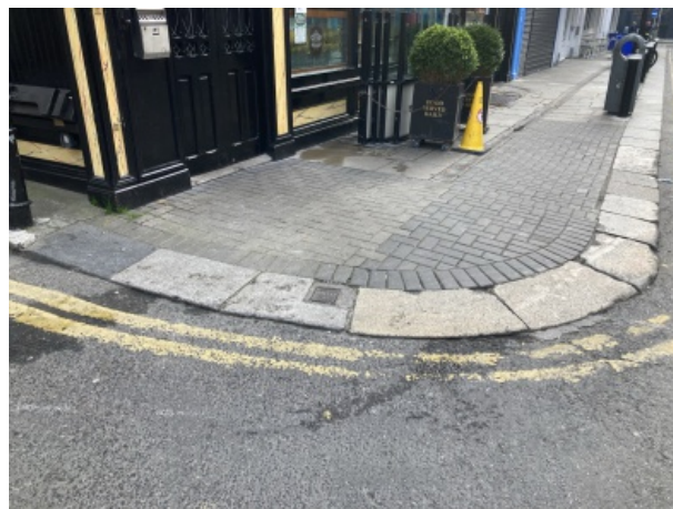
Feature Number: 17 - Historical granite kerbstone mixed with modern replacement kerbstones on the corner of 8-9 Duke Street and Duke Lane.
