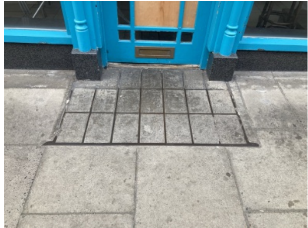
Feature Number: 13 - Cast iron access cover with concrete inserts/ previous light well cover, 13 Duke Street
