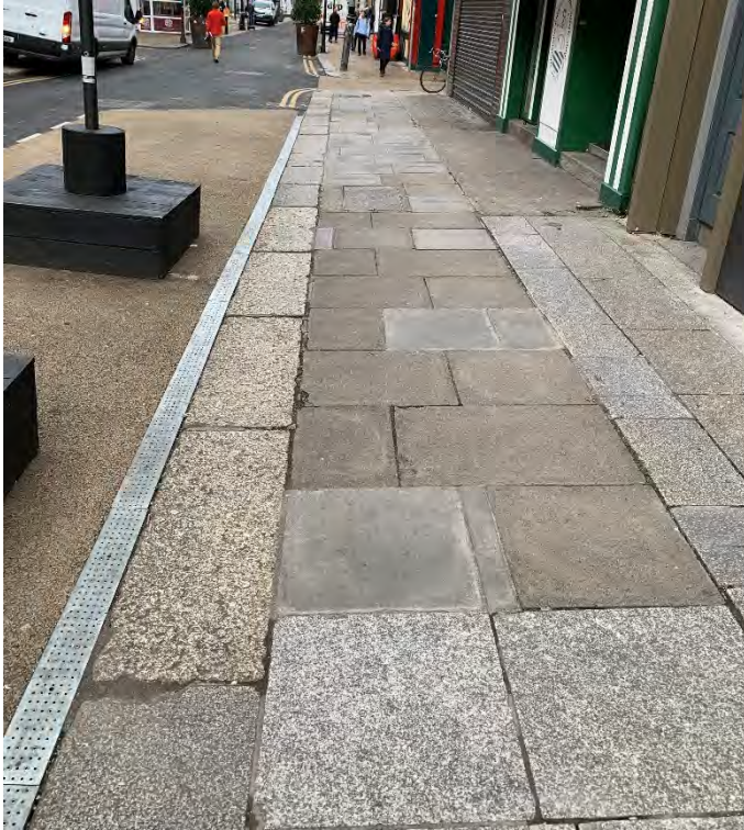
55. Photograph of typical example of historic Leinster Granite kerbstones with modern concrete pavers along eastern end of north footpath (outside Antony Peto, 14 Anne St S / Isabelle's, 13-14 Anne St S)
