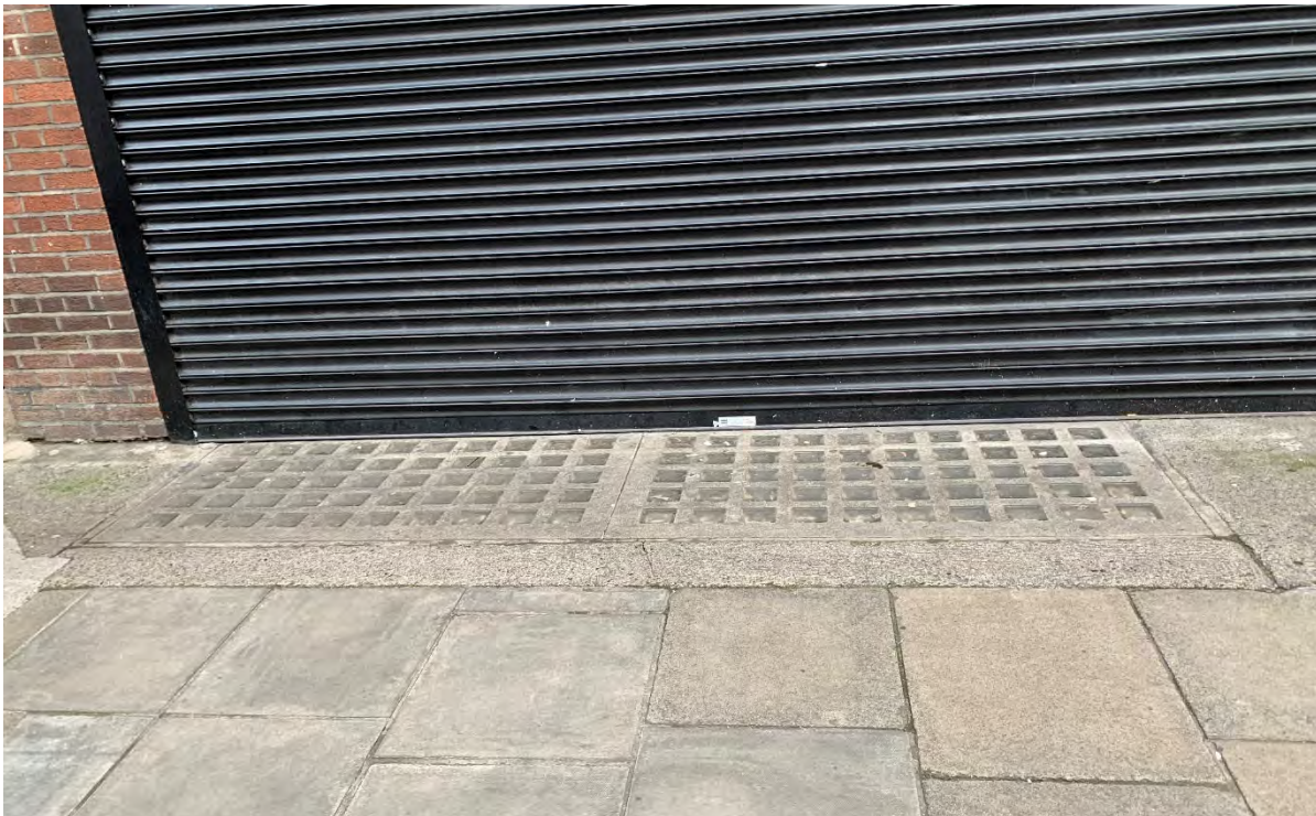
56. Photograph of modern concrete pavement light with modern poured concrete surrounding, outside vacant unit.
