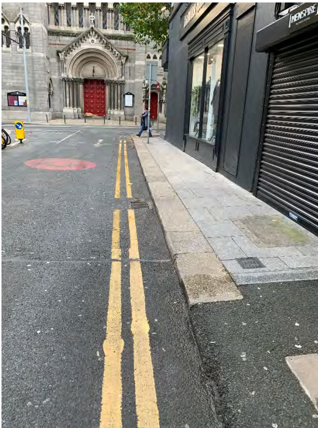
47. Photograph of historic Leinster granite kerbstones outside vacant unit and James Herren (44 Dawson St).
