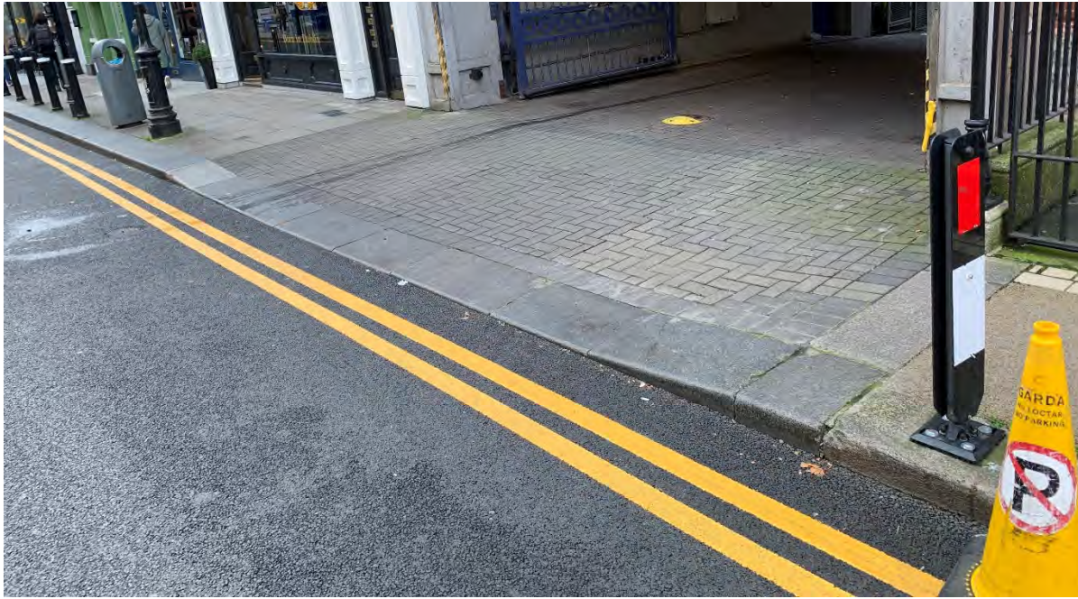
8. Photograph of dished kerb to vehicle entrance next to Duke St Gallery (17 Duke Street). Modern materials.
