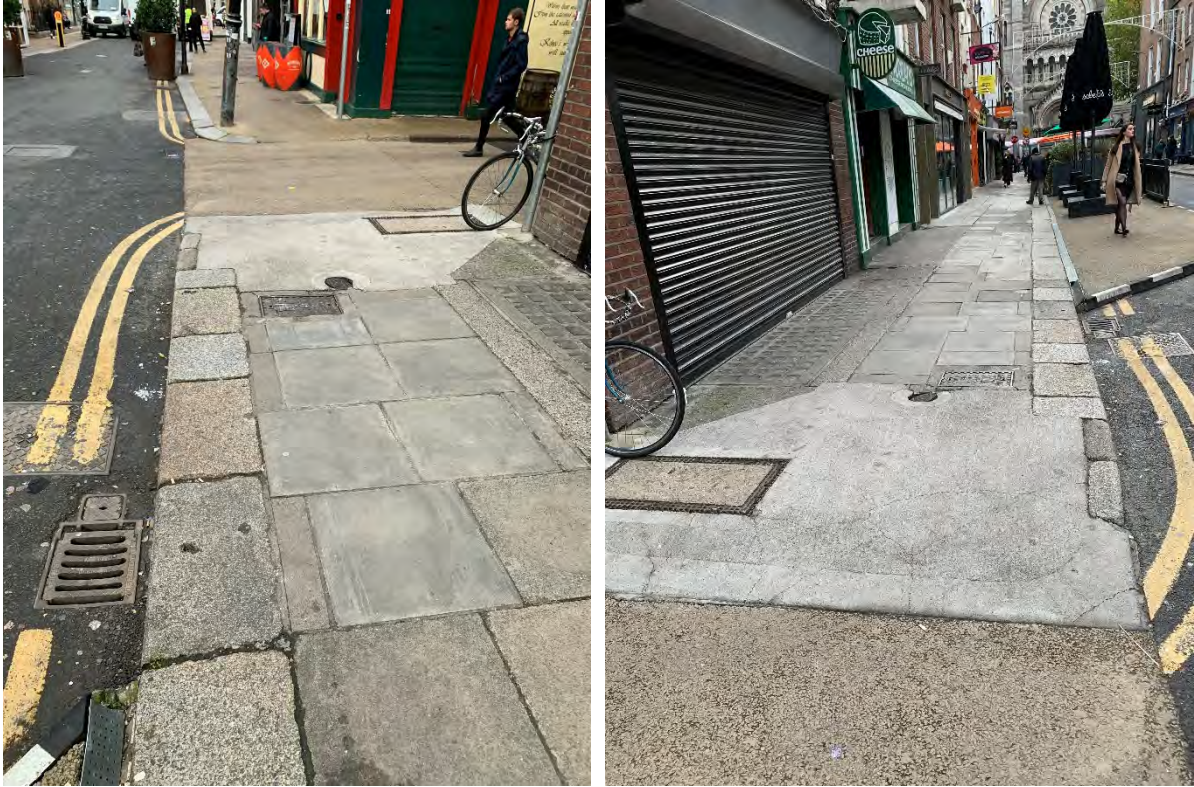
57 & 58. Photograph of historic Leinster Granite kerbstones stop at eastern corner junction with Duke Lane Upper, note two 'slim' historic kerbstones before radius – presumably cut in past
