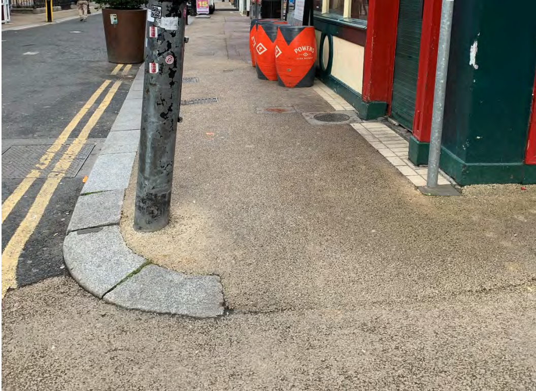
59. Photograph of good quality kerbstones at western corner junction with Duke Lane Upper. Modern kerbstones beyond.
