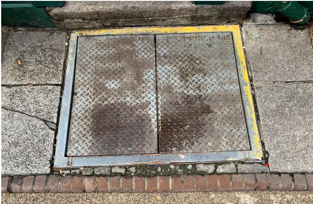
29. Photograph of modern metal keg-drop / cellar cover outside side entrance to John Keoghs (9 Anne St S), off Duke Lane Upper. Historic Leinster Granite edge pavers to two sides.
