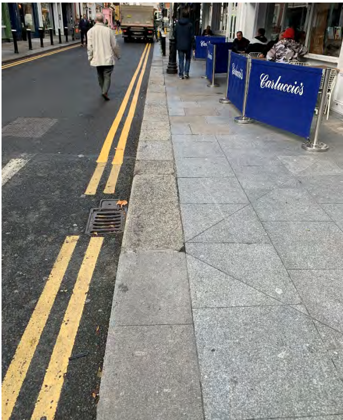
18. Photograph of historic Leinster granite kerbstones and junction with modern kerbstones at dished pedestrian crossing outside Carluccio's restaurant (52 Dawson Street) / Dawson Street footpath
