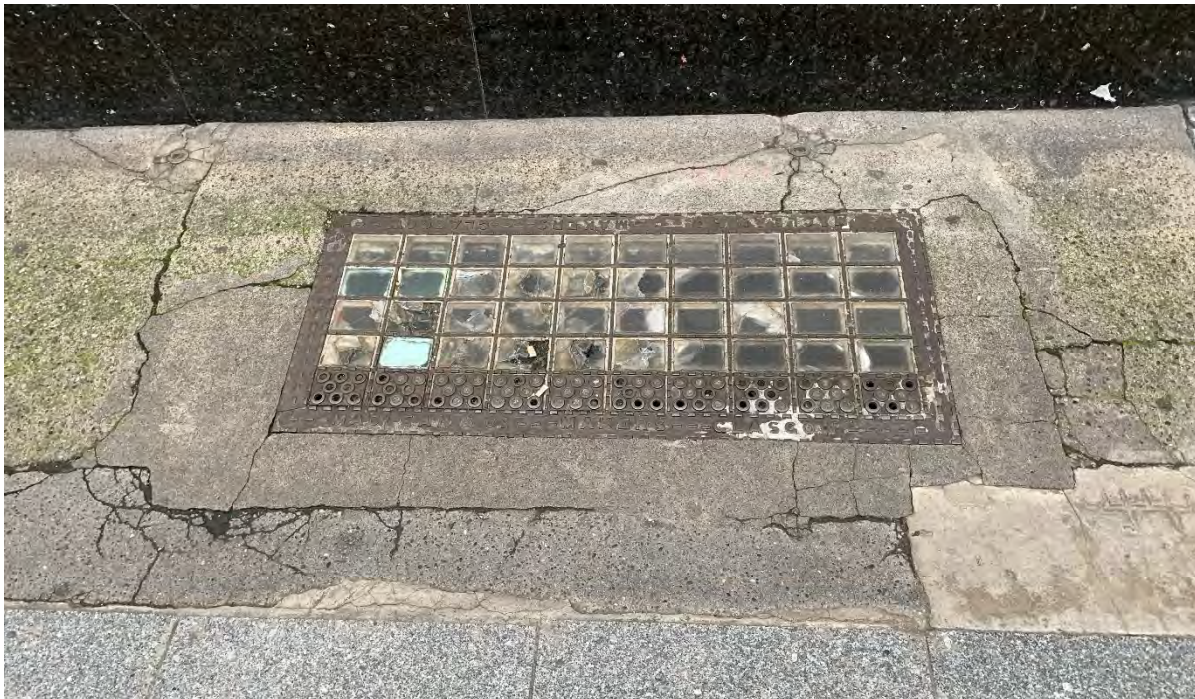
51. Photograph of historic cast iron pavement light with modern poured concrete footpath adjacent, outside Abrahams Tailors (17 Anne St S).
