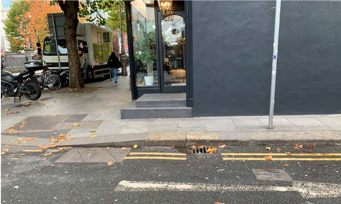
48. Photograph of historic Leinster granite kerbstones and junction with modern kerbstones at dished pedestrian crossing outside James Herren (4 Dawson St) / Dawson Street footpath.
