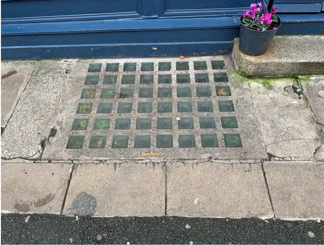
46. Photograph of historic Leinster granite edge paver (1 no to left of pavement light), as mentioned above outside Deirdre O'Donnell jeweller (19 Anne St S).
