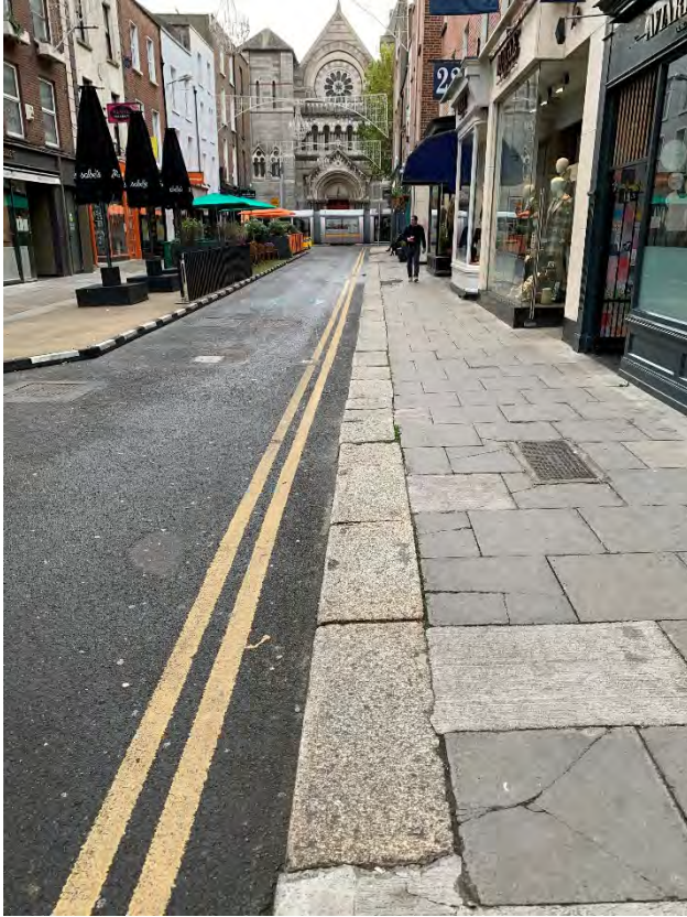
42. Photograph of run of historic Leinster granite kerbstone on eastern end of south footpath, from Links London (25-26 Anne St S) to James Herren (44 Dawson St). Note two asphalt repairs in middle and background.
