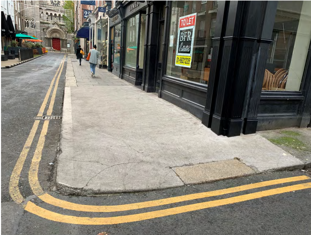
37. Photograph of corner of Anne Street South and Anne's Lane on eastern side, badly damaged in past with unsightly asphalt repairs. One historic Leinster granite kerbstone visible to right of image. (see image & note below)
