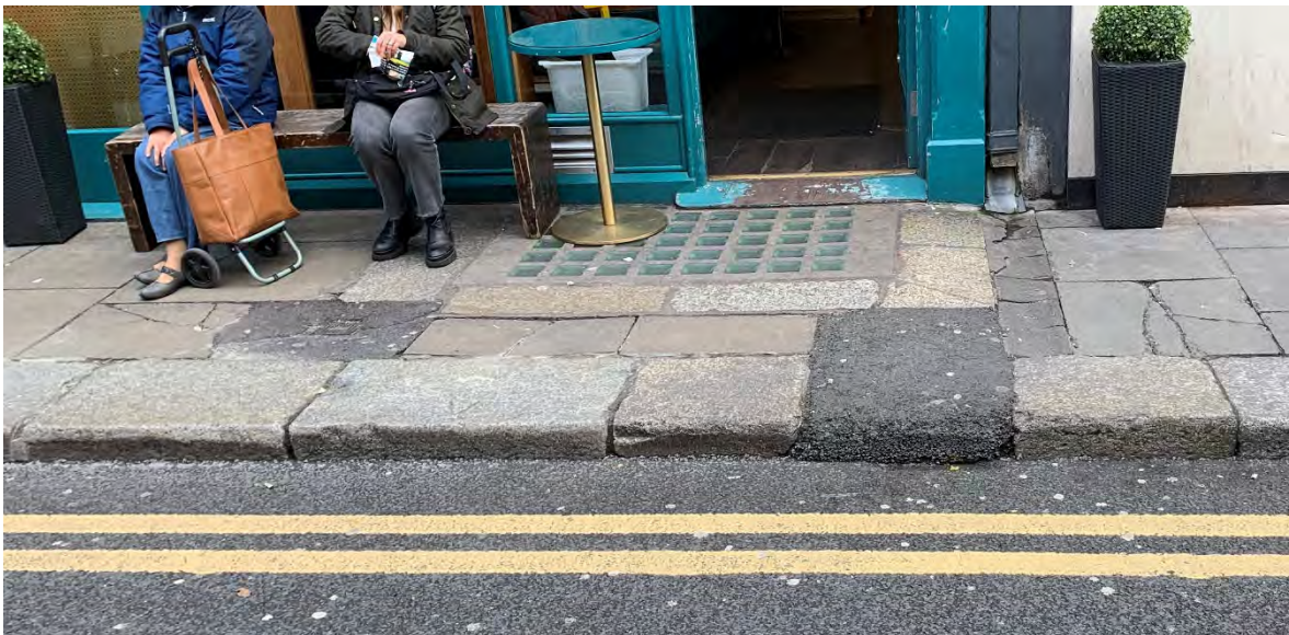
43. Photograph of section of footpath outside Dolce Sicily (20 Anne St S), including modern concrete pavement light with historic Leinster granite edging pavers and historic Leinster granite kerbstones. Also, poor asphalt repairs to kerbstones and footpath.
