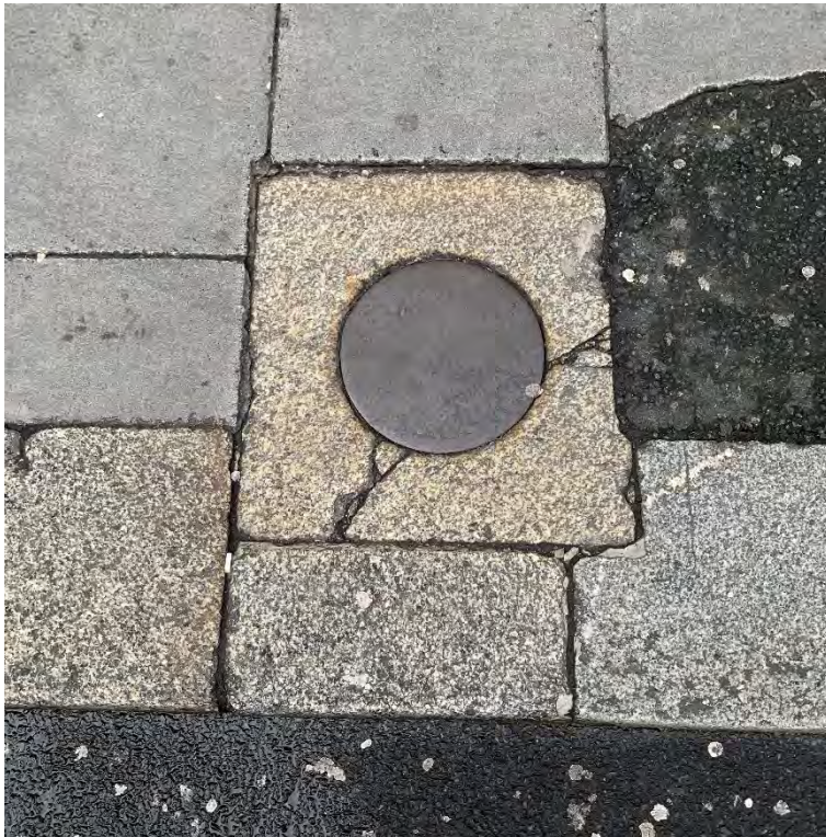
41. Photograph of historic coal hole cover set in historic Leinster Granite paver outside Monaghans Cashmere (21 Anne St S)
