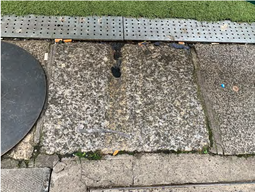
54. Photograph of example of dished channels in historic Leinster Granite kerbstones along eastern end of north footpath (note these do not align with party lines of adjacent properties which would suggest that they have been repositioned at some time in the past)
