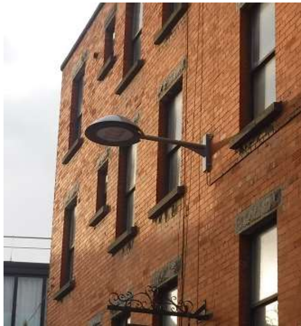
Fig 7: Wall mounted public light fitting
