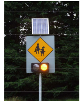
SCHOOL AHEAD SIGN WITH FLASHING AMBER BEACONS
