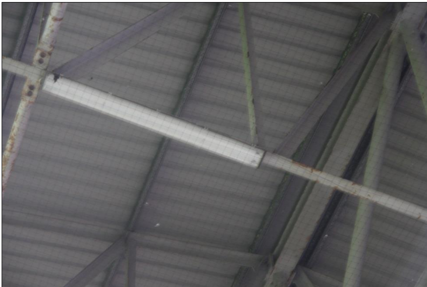
Plate 8 Netting on the RSJ in Jodi Stand to deter nesting birds. Would also discourage roosting bats as they would not have a clear flight path.
