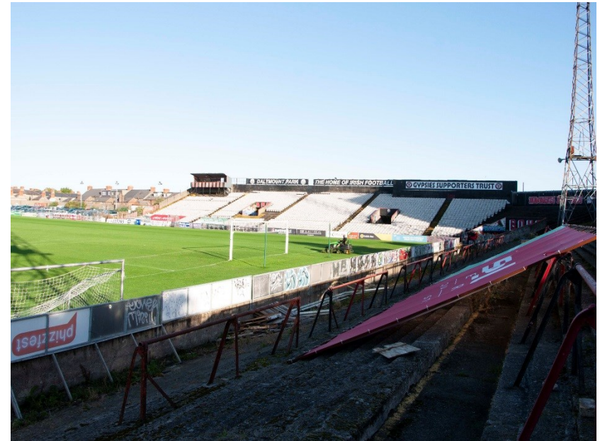
Plate 6: View of Connaught St. showing Stand, showing crush barrier, from the Tramway End stand, facing northwest.
