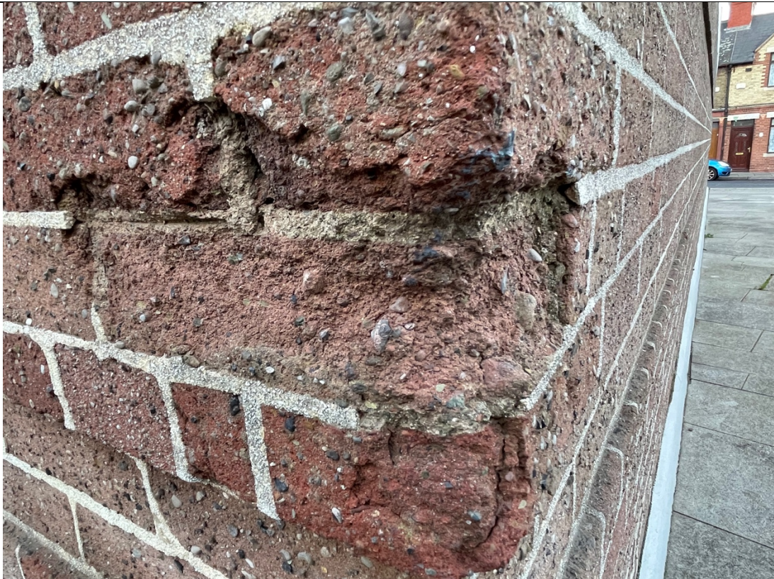
10. - Detail to corner of above location, evidencing deteriorated brick condition
