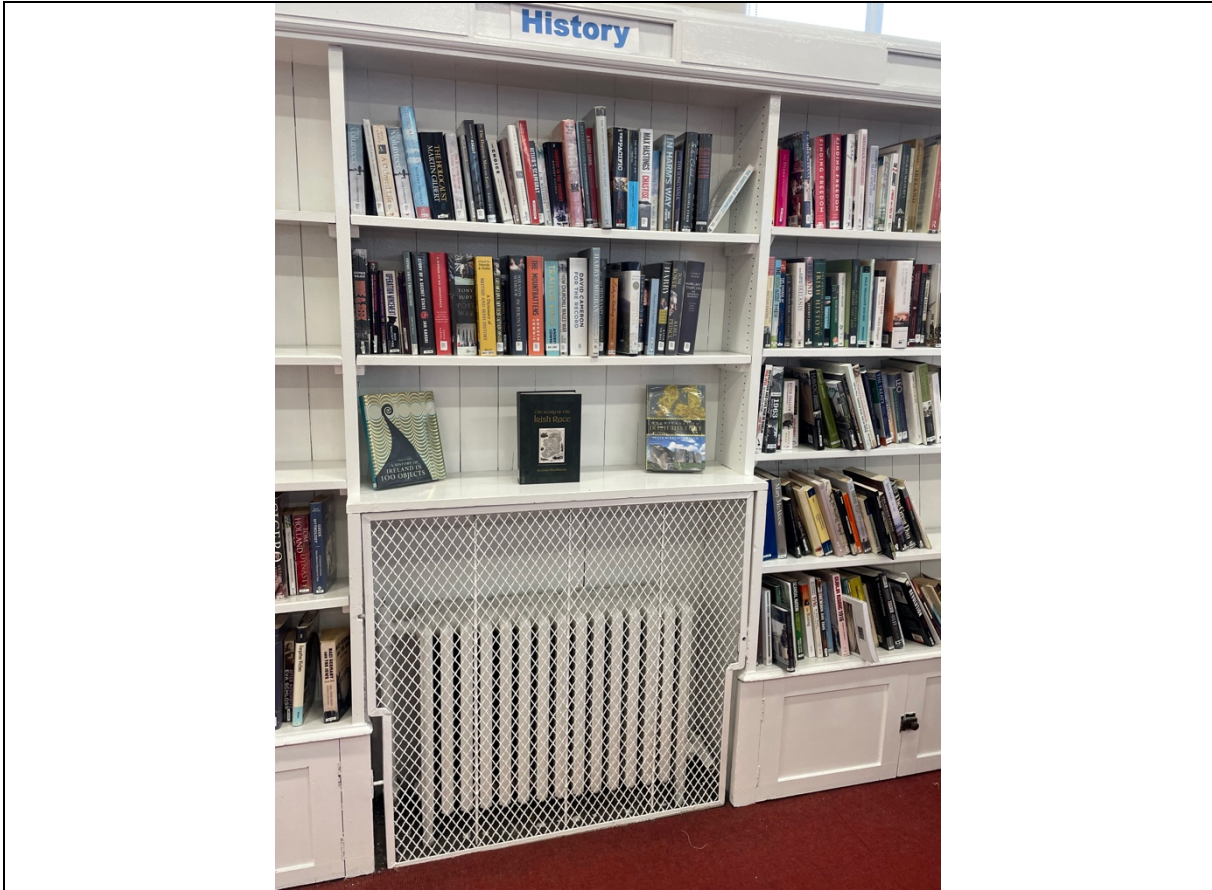
31 – Detail of radiator recessed to shelving walls
