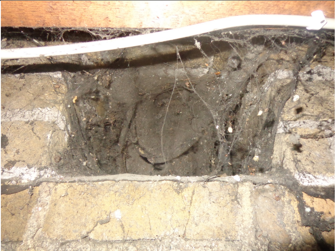
41 - Ditto. Note proliferation of cobwebs evidencing the absence of sufficient ventilation
