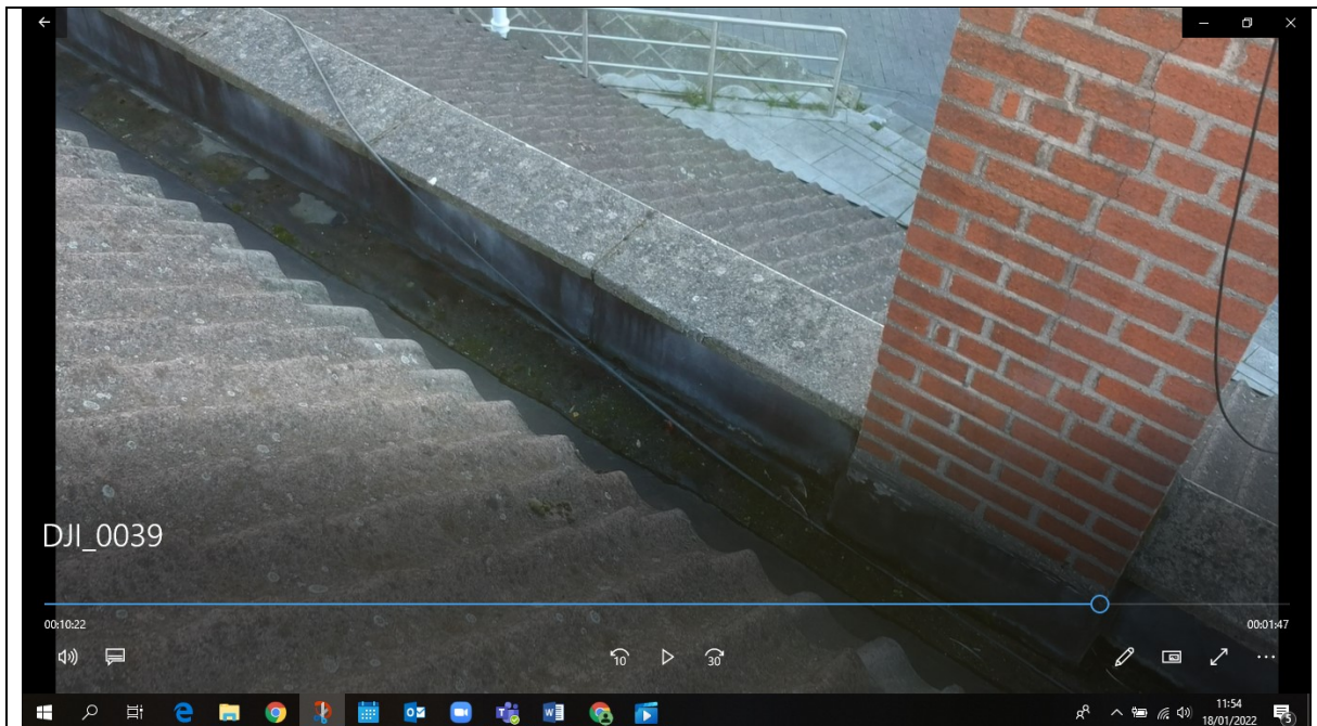
23. - View of vertical hairline cracking to front side of chimneystack
