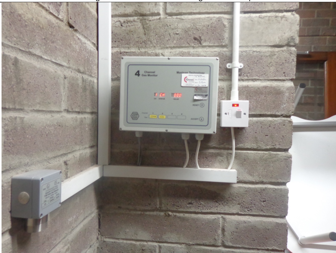
50 - View of gas detection equipment in rear plant room
