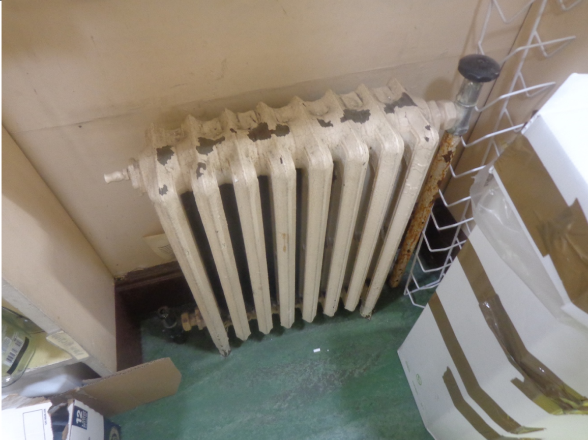
46 - View of typical columnar radiator (in rear lean-to)
