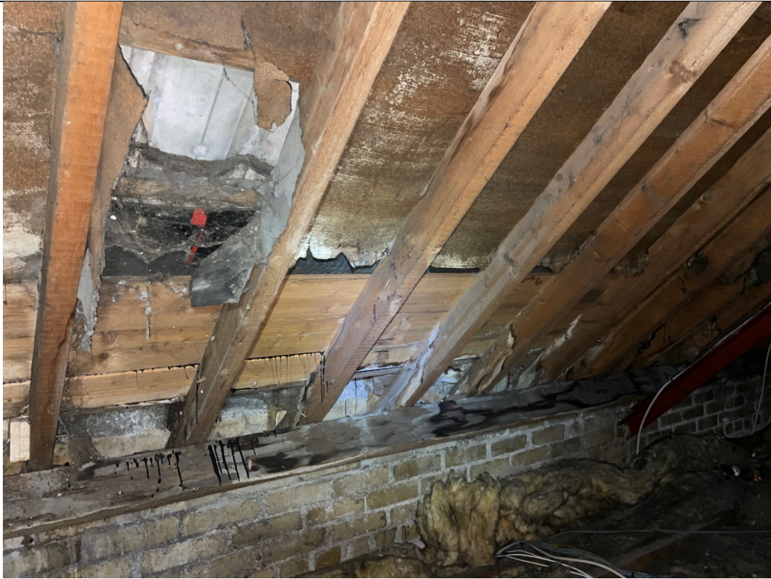
53 – Typical damage to roof underlay above parapet level &
