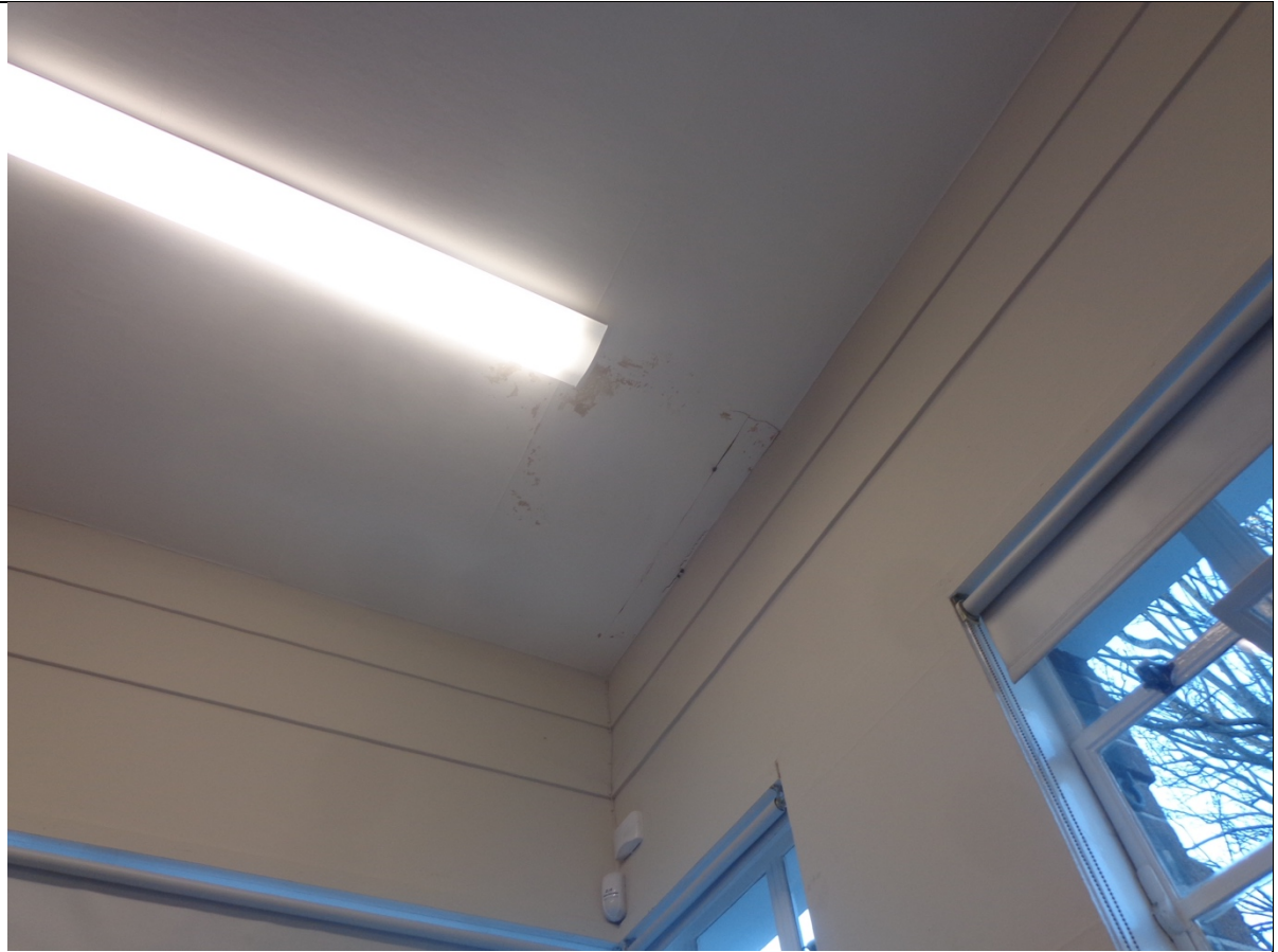
33 - View of water ingress in extreme rear right corner
