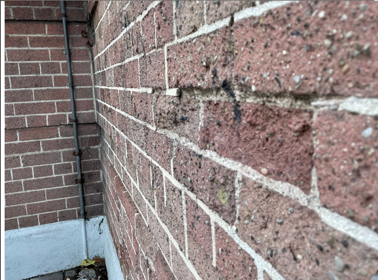
11. – Detail to above location, evidencing deteriorated brick condition
