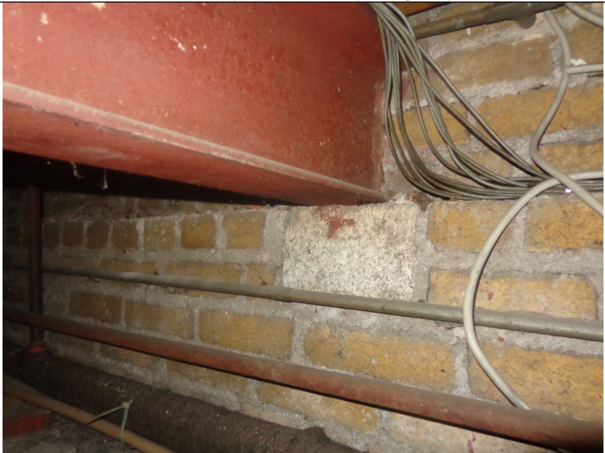
38 - View of granite padstone built into external wall base and supporting bearing end of steel beam
