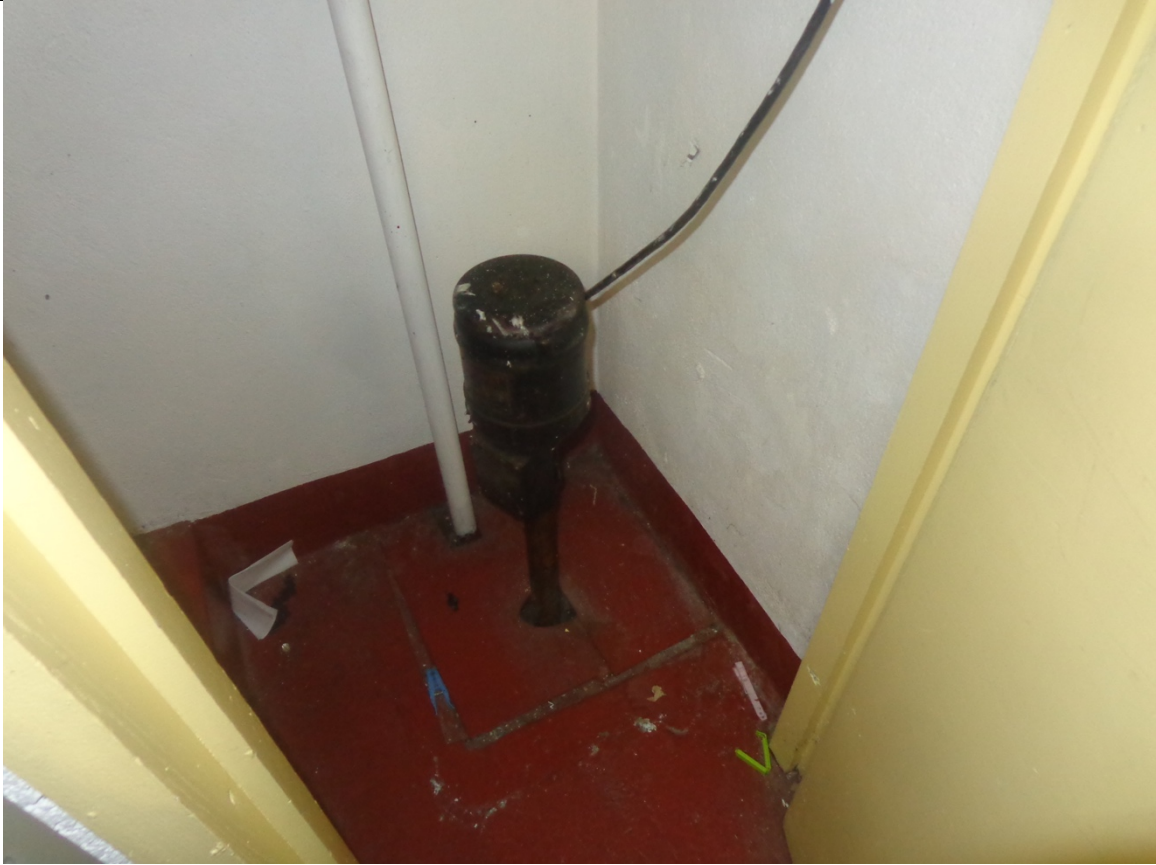
45 - View of sump pump at bottom of basement stairs
