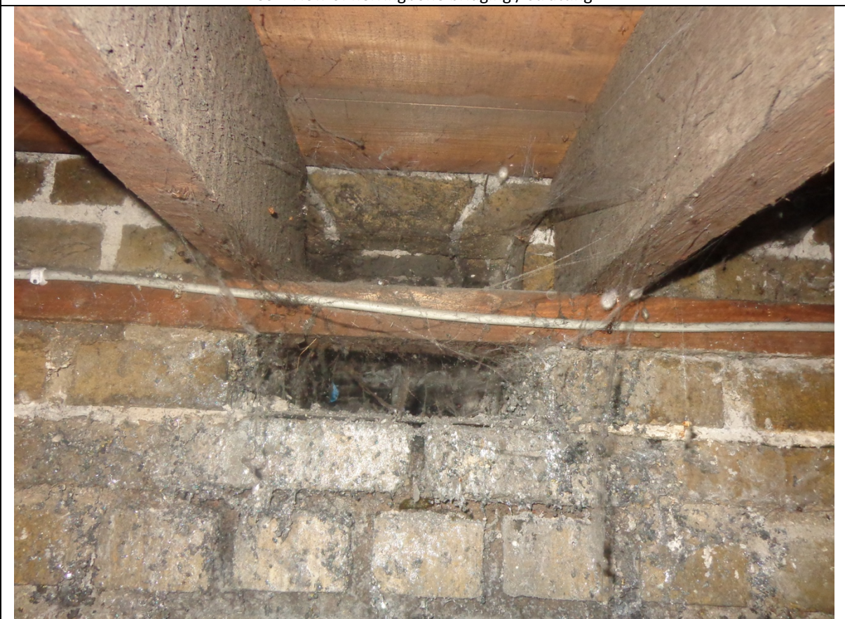
40 - View of original opening to accommodate subfloor vent at base of external wall
