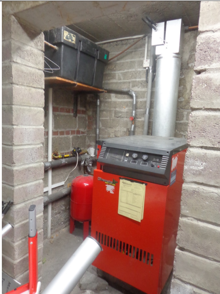
49 - View of gas boiler and cold water storage tank in rear plant room
