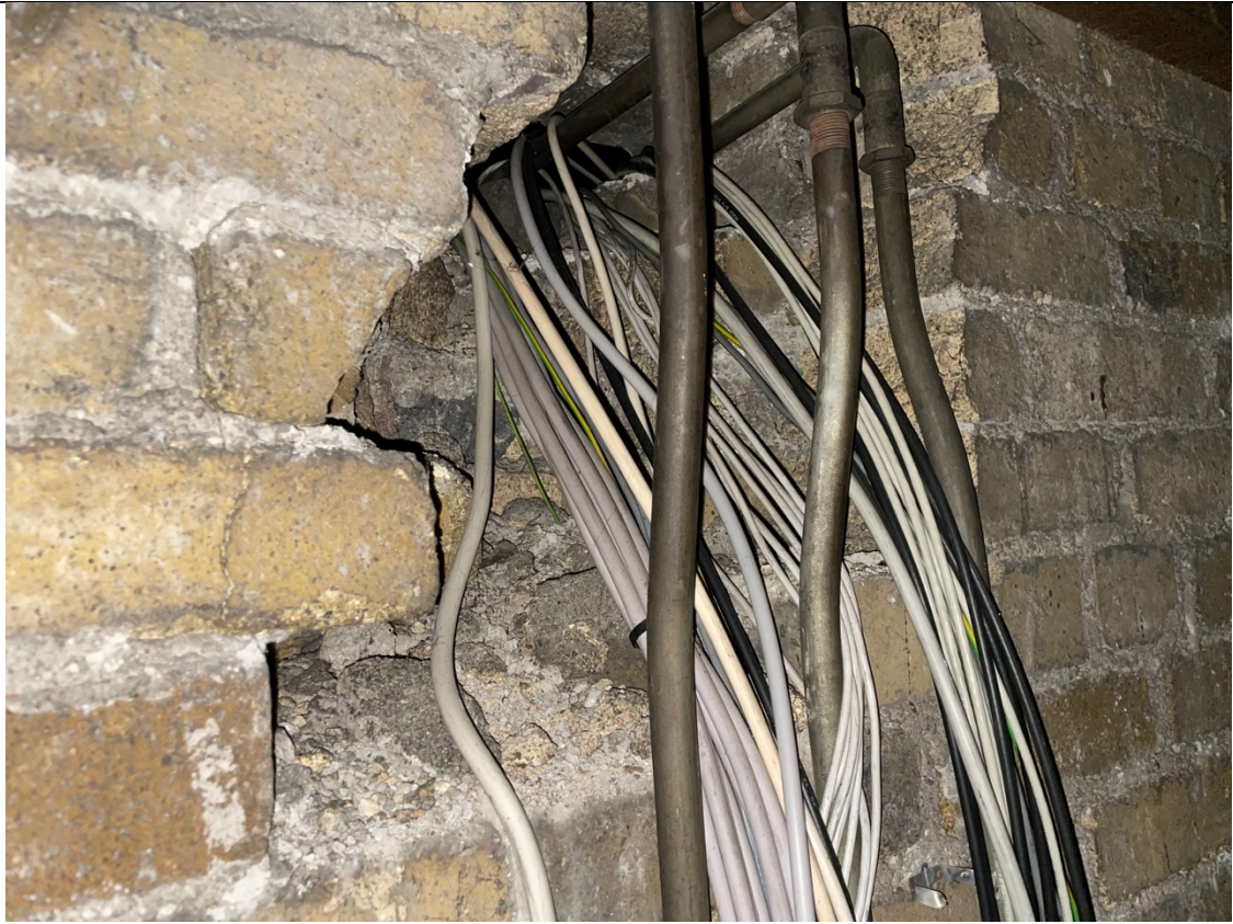
35 – Detail of services opening in rear wall between main attic and lean-to attic illustrating solid concrete brick construction of external walls
