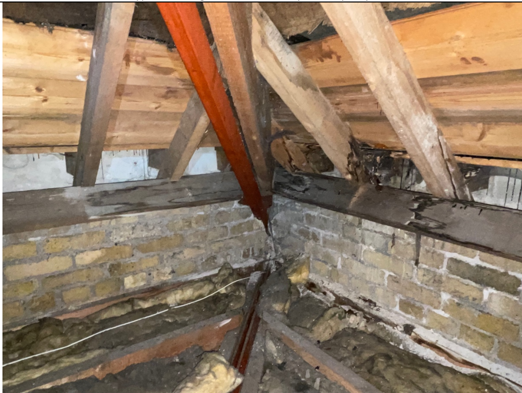
54 – Detail at corner & water ingress staining to lower purlin
