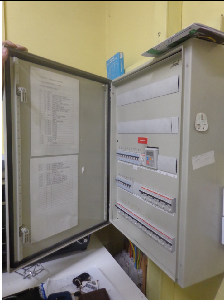
47 - View of electrical distribution board (in rear lean-to)
