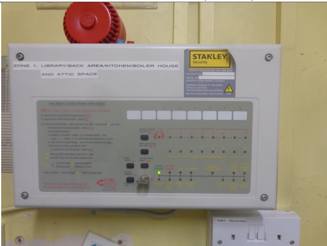
48 - View of addressable fire alarm control panel (in rear lean-to)
