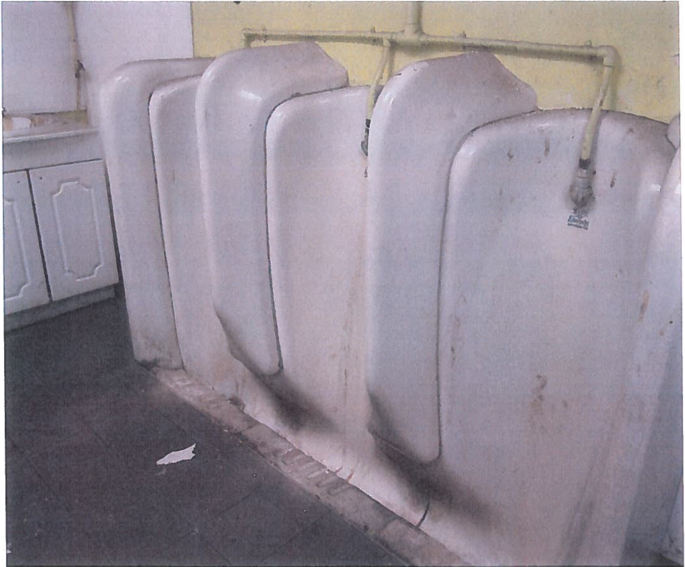
Fig 55 Ceramic urinals in men's toilets
