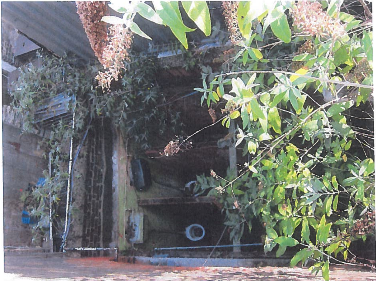
Figs 46 Derelict toilets viewed from roof
