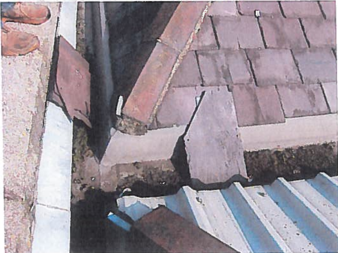
Figs 78 & 79 Roof slates slipping and flashings require
