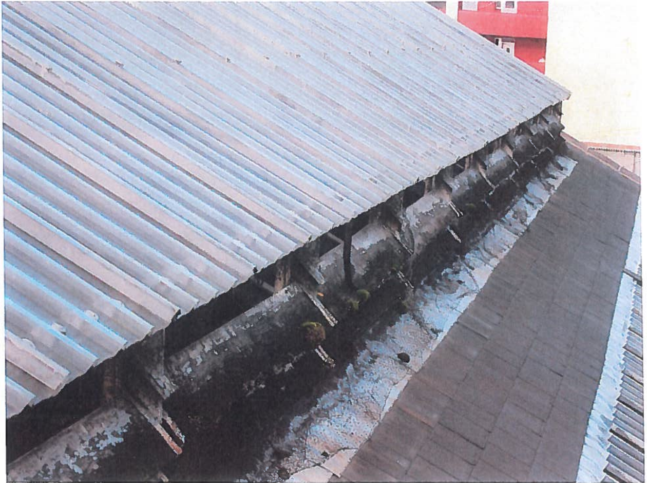
Fig 84 Louvres of lantern providing ventilation
