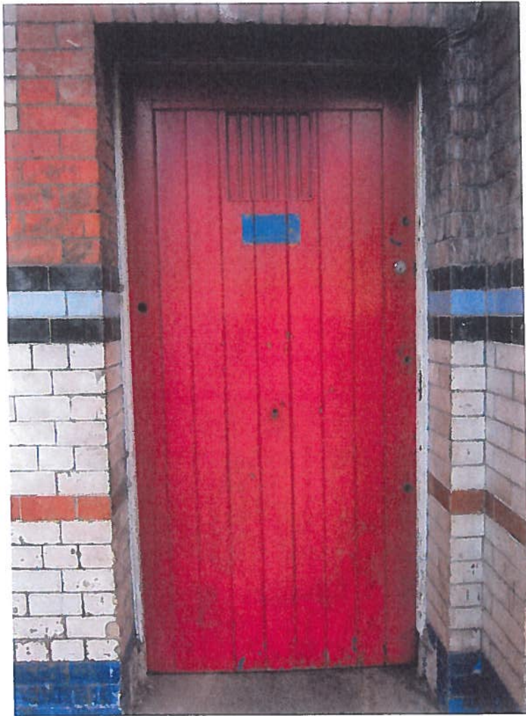
Fig 67 The original sheeted internal doors have survived generally. The tall oak gates are replacement with the original wrought iron reinstated.
