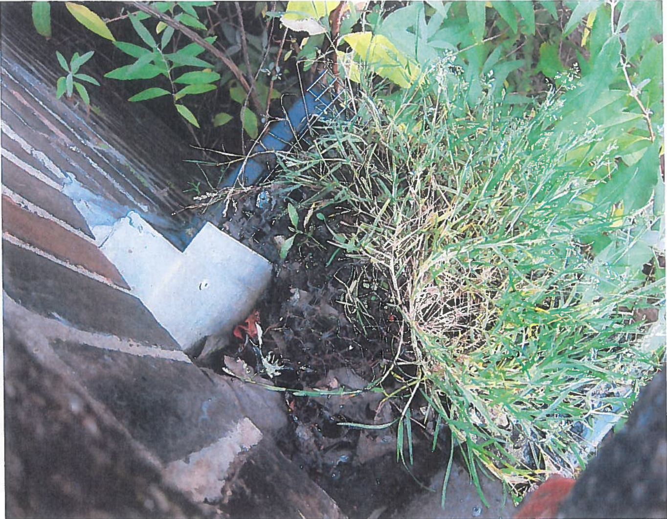
Fig 87 Blocked up rainwater outlets
