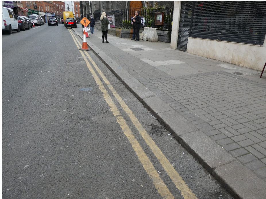
Figure 12: Pavement on east side of street south of St. Catherine's Church
