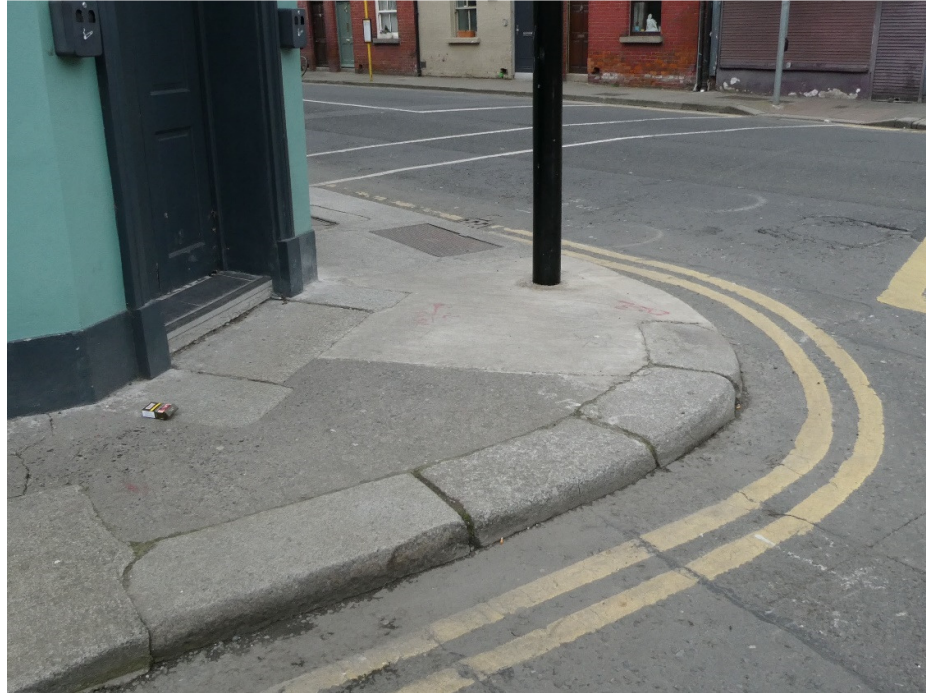
Figure 29: Corner to south-west of junction with The Coombe with stone threshold to pub
