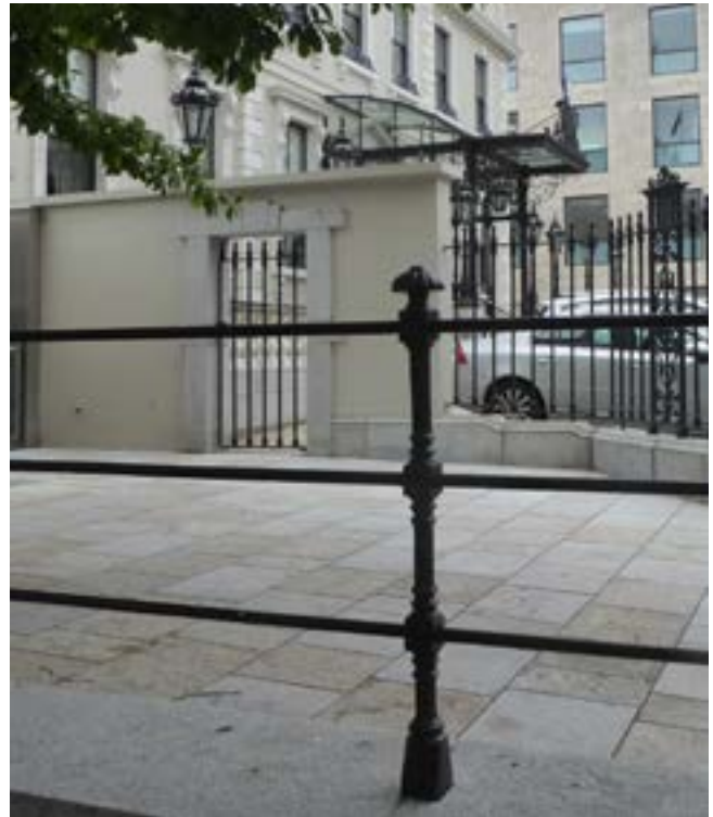
Fig. 4.15 Existing Cast Iron post at southern edge of Garden. These posts will be removed and will be re-laid at the new lower level.
