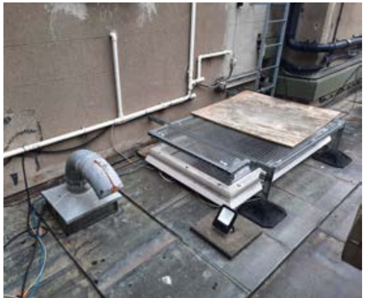
Fig. 4.50 Existing (unused) rooflight to toilets to be removed
