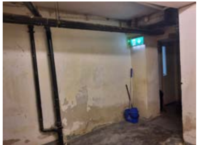
Fig. 4.40 Southern internal wall of basement where an opening is to be made for the lift insertion
