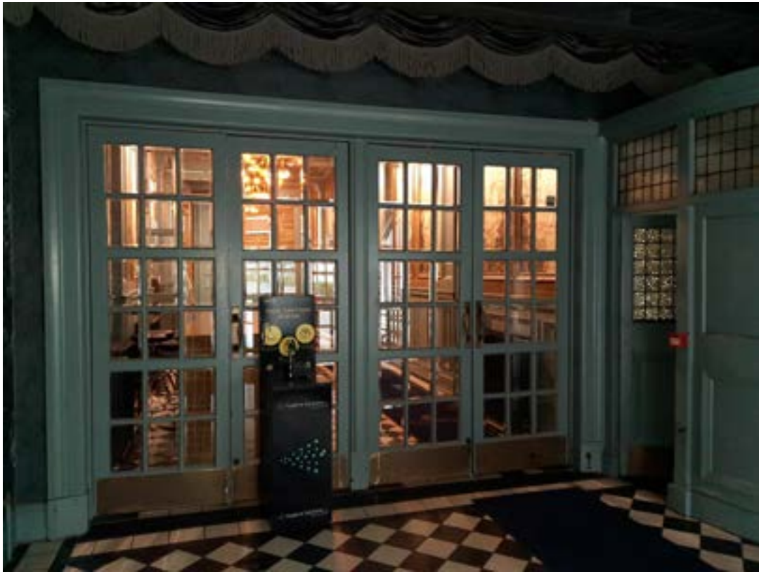
Fig. 4.24 Existing lobby doors inside main entrance of Entrance Vestibule. Ticket booth located to RHS of image
