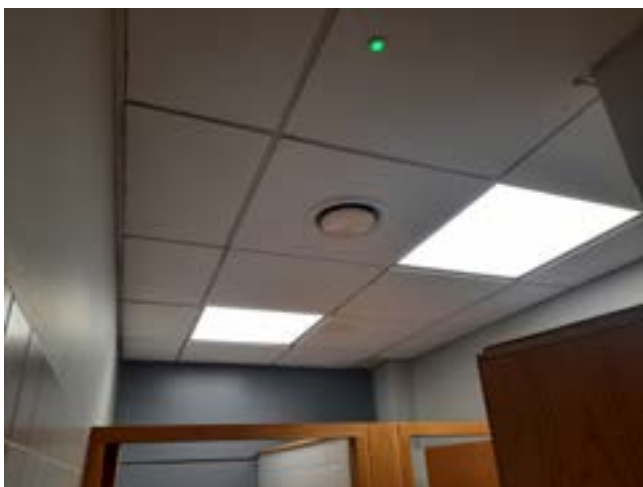
Fig. 4.43 Modern suspended ceilings located in the existing toilets adjacent to the Rear Hall
