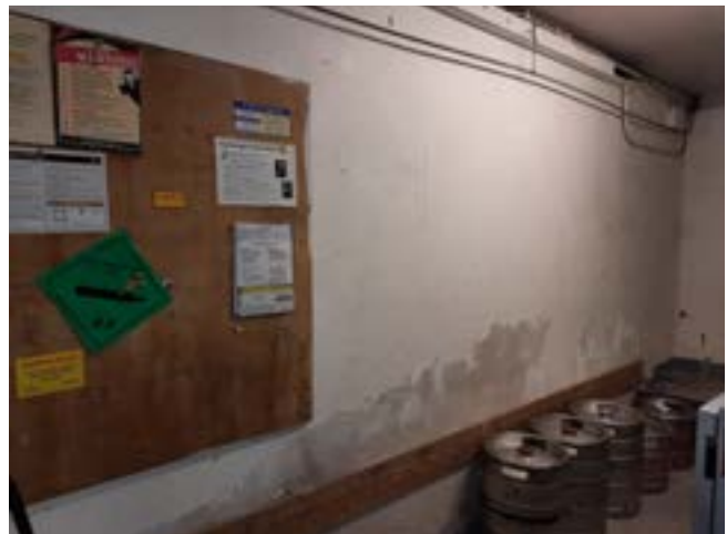
Fig. 4.41 Northern internal wall of basement where an opening is to be made for the lift insertion
