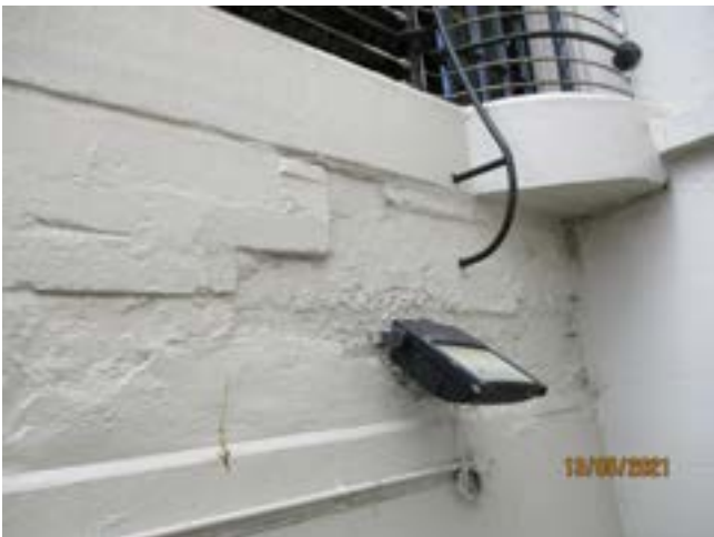
Fig. 4.9 Upper section of wall to light well is of concrete. Lower section is of stone.
