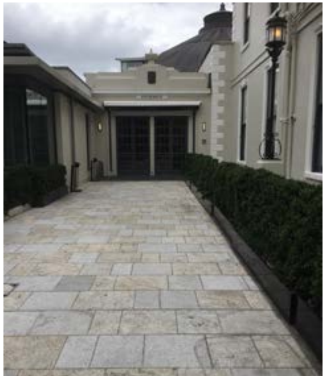
Fig. 3.27: Modern paving laid to upper part of Approach Route to Supper Room Entrance Vestibule
