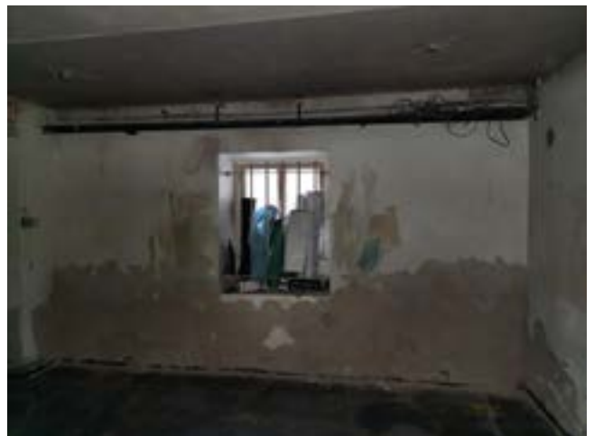
Fig. 4.36 Northern external wall of basement where the new door insertion is to take place
