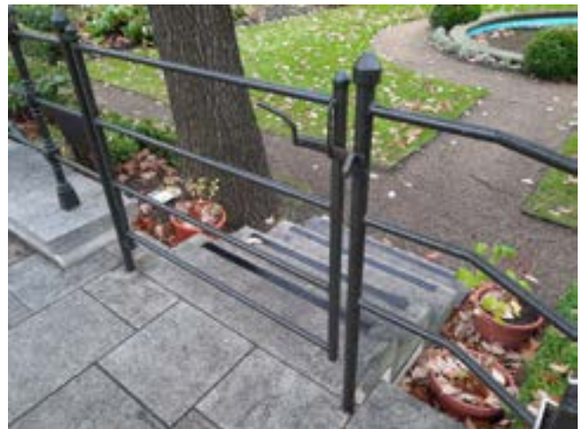
Fig. 4.6 Modern gate and railing between the Lord Mayor's Garden and approach route to the Round Room. All modern paving throughout.
