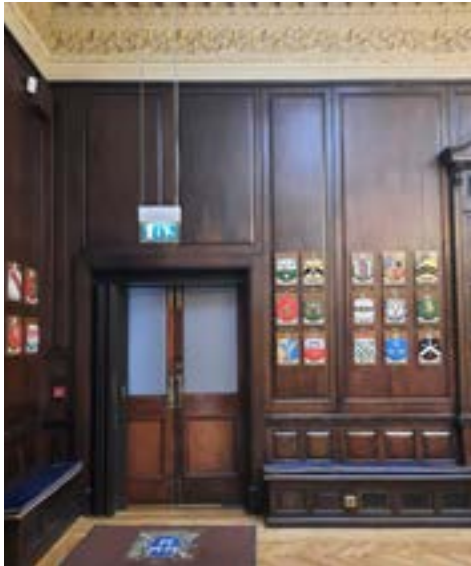
Fig. 4.53 Doors to Entrance Vestibule to be blocked up and clad in Oak panelling which will be taken from opposite end.
