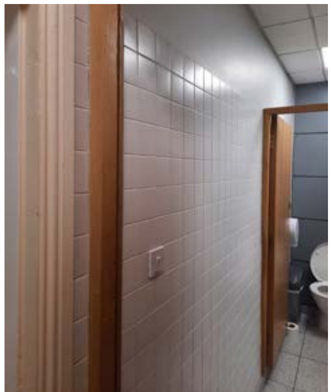
Fig. 4.45 Modern tiled wall located in the existing toilets adjacent to the Rear Hall
