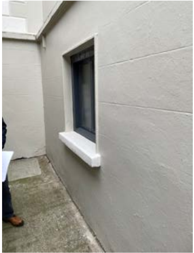
Fig. 4.10 Window to be converted to doorway located along basement northern wall of Mansion House.
