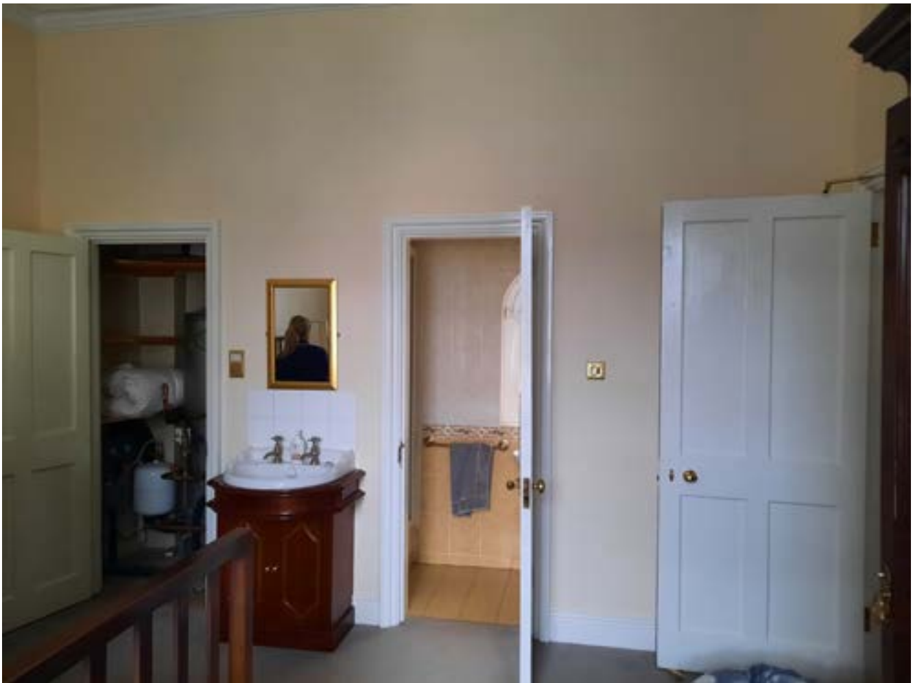
Fig. 4.47 Existing southern wall to the Mansion House, First Floor bedroom. En-suite to be removed to allow for lift access.
