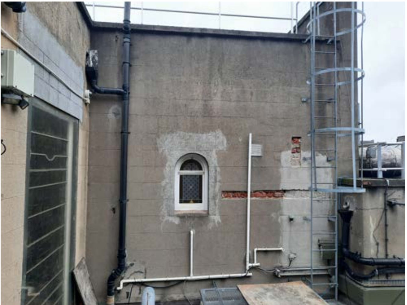
Fig. 4.48 External south facing wall to be modified to allow for provision of lift access door and door access between first floor and external space. Note section of modern block infill is present along the wall. (RHS image)
