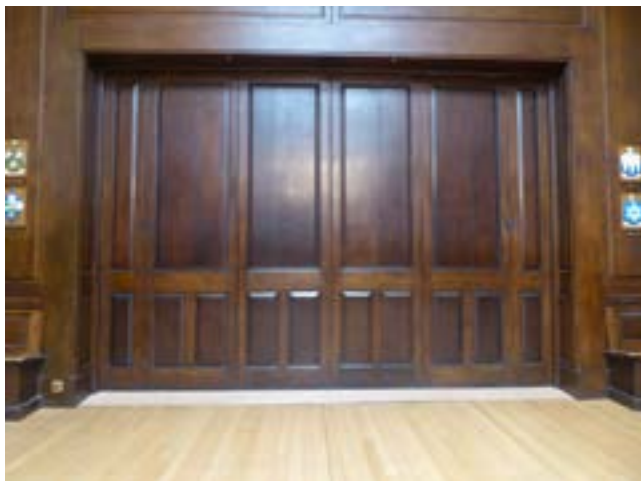
Fig. 3.38 Oak folding doors installed to western wall of Oak Room, leading to the adjacent Drawing Room
