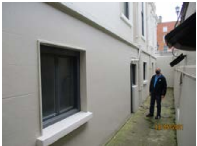
Fig. 4.11 Window (LHS of Image) to be converted to doorway located along basement wall.
