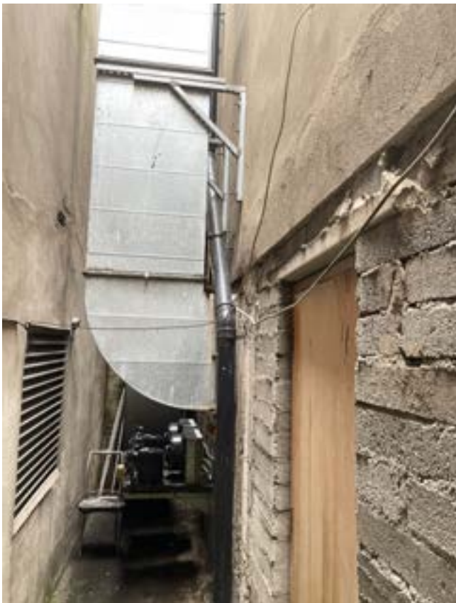
Fig. 4.63 Basement level of light well looking west. Boiler Room to Mansion House LHS of images.
