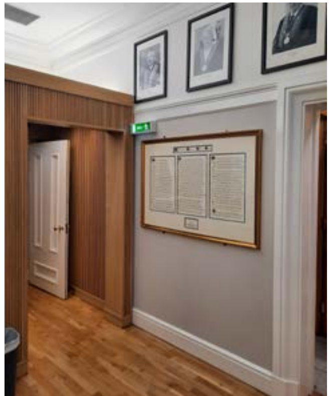
Fig. 4.44 Existing original wall located in the Rear Hall of the Ground Floor to the Mansion House. Wall to be altered to accommodate provision of Lift.
