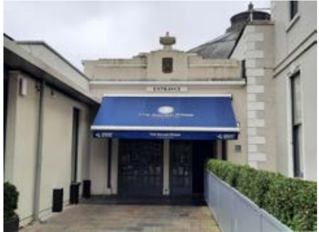
Fig. 4.2 The single-storey 1928 masonry elevation generally appears to be in reasonably good condition. The modern canopy hides much of the architectural detail.
