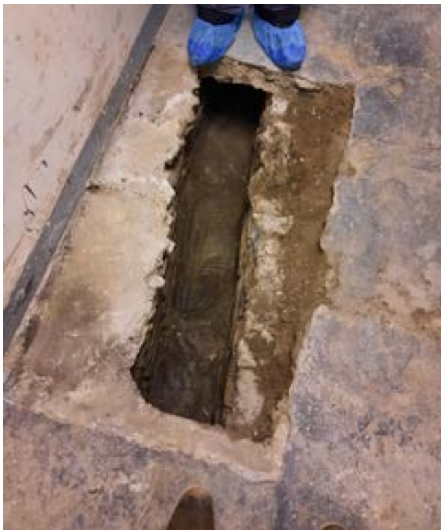
Fig. 4.39 Stone flags lifted in the basement floor at the location of the proposed lift pit
