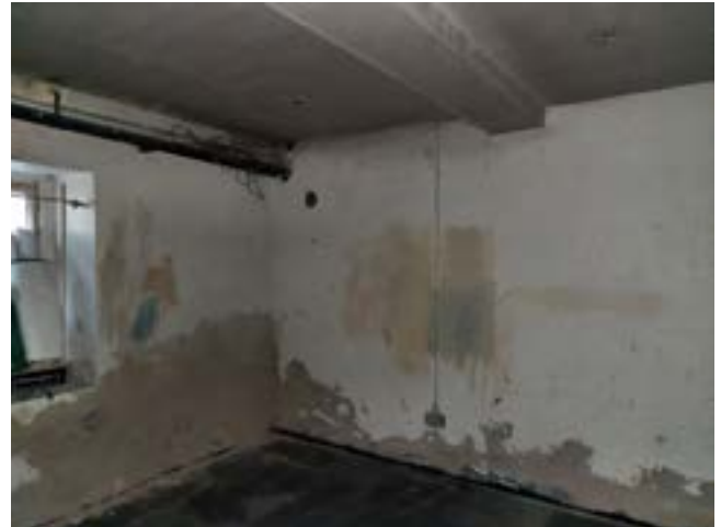
Fig. 4.35 Eastern internal wall of basement where an internal door opening is to be made to adjacent room
