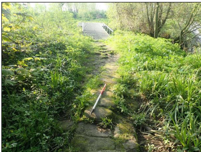
Plate 22: Existing footbridge proposed to be removed; baffle rests to the left of this bridge (1m scale).
