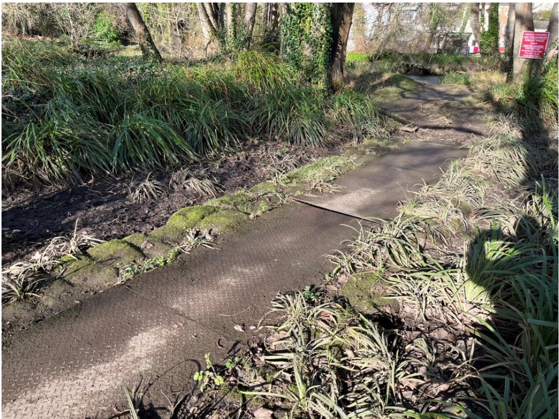
Photo 4: Section of the steel walkway that is required to be removed prior to the construction of the new walkway.
