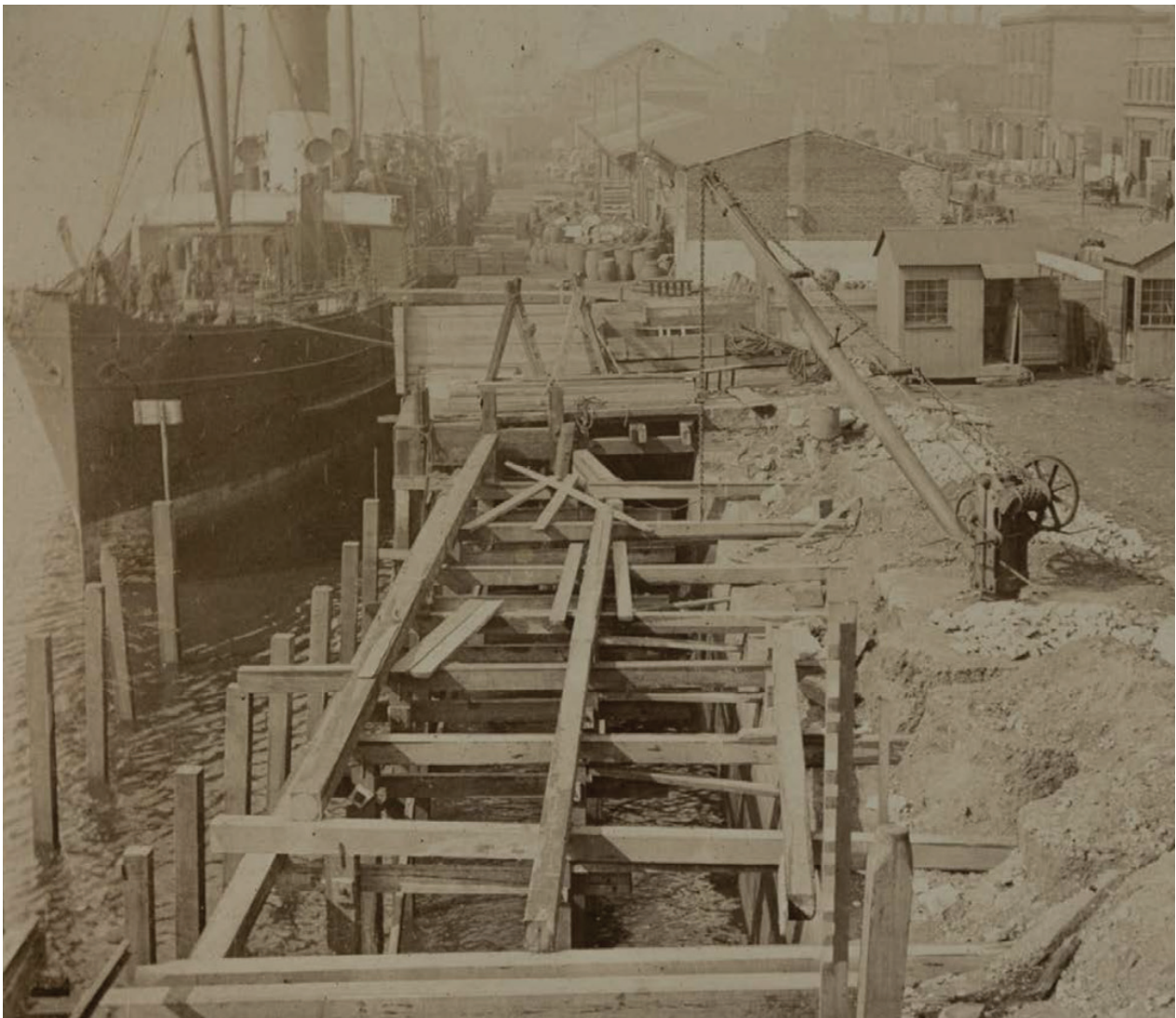
Figure 18 - Reconstruction of part of North Wall quays to provide deeper water berths c.1905 (DPA)
