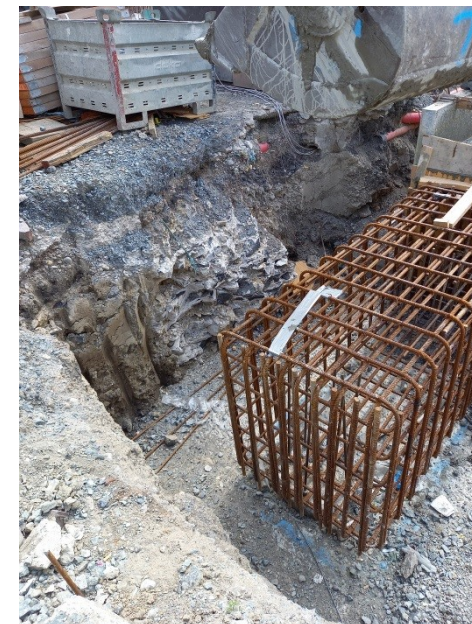
Plate 23: Northern wall of Portobello Harbour, as exposed on the site of the future hotel, adjacent and to the west.
