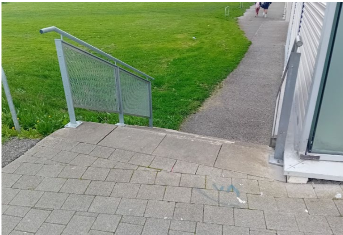
Figure 8.4 – Existing Steps with no Tactile Paving
