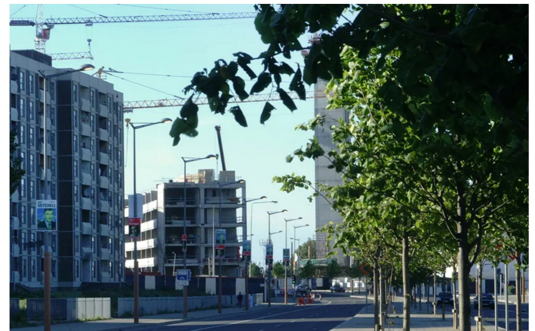
Image 17 - Construction of Santry Cross underway on available open lands adjacent to existing spine block of flats- View looking north along Ballymun Road, what is now Site 5.
