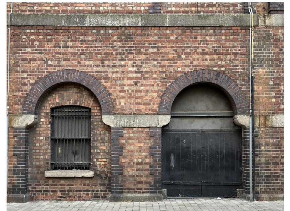
Figure 68: Materials in the surrounding context
