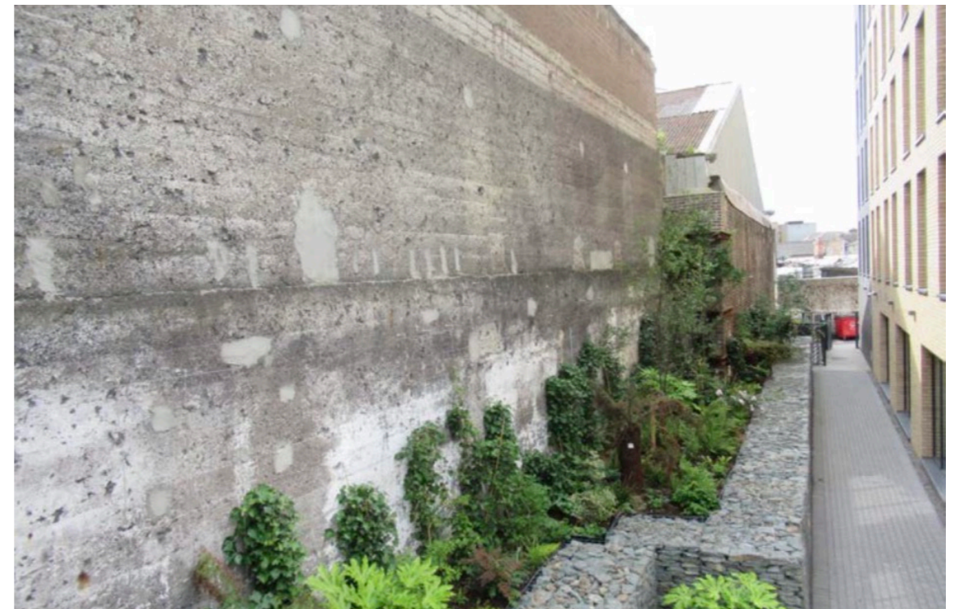
Above: Existing historic boundary wall, as viewed from neighbouring side, to be protected.
