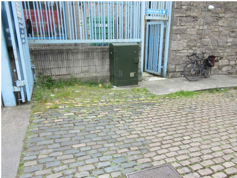
Plate No. 16. Detail view showing evidence of changes to the the original stone setts at the north end of Stanley Street. Different types of stone, of different colours, can be seen. Most of the setts are pinkish granite, with black basalt stones seen in other areas such as above. The proposed extension of the public footpath on the east and west edges of Stanley Street, will improve accessibility into the new development.
