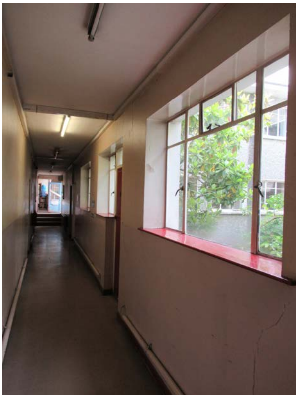
Plates No. 24 and 25. General internal view looking down the internal corridors in the mid-20 th century offices. The steel windows are notable but also quite typical of mid-20 th century Irish commercial structures. Otherwise there is nothing remarkable in the design or construction of this structure.
