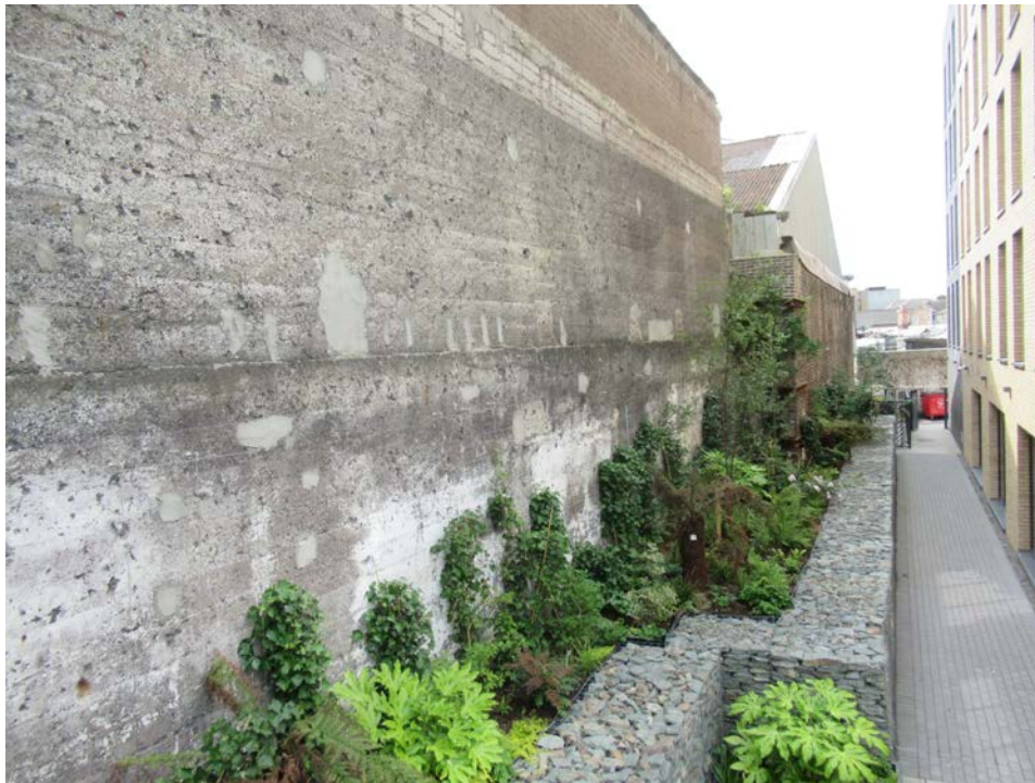
Plate No. 41. General view looking south, showing concrete boundary wall along the northern end of the west site boundary as it appears from the adjacent site.
