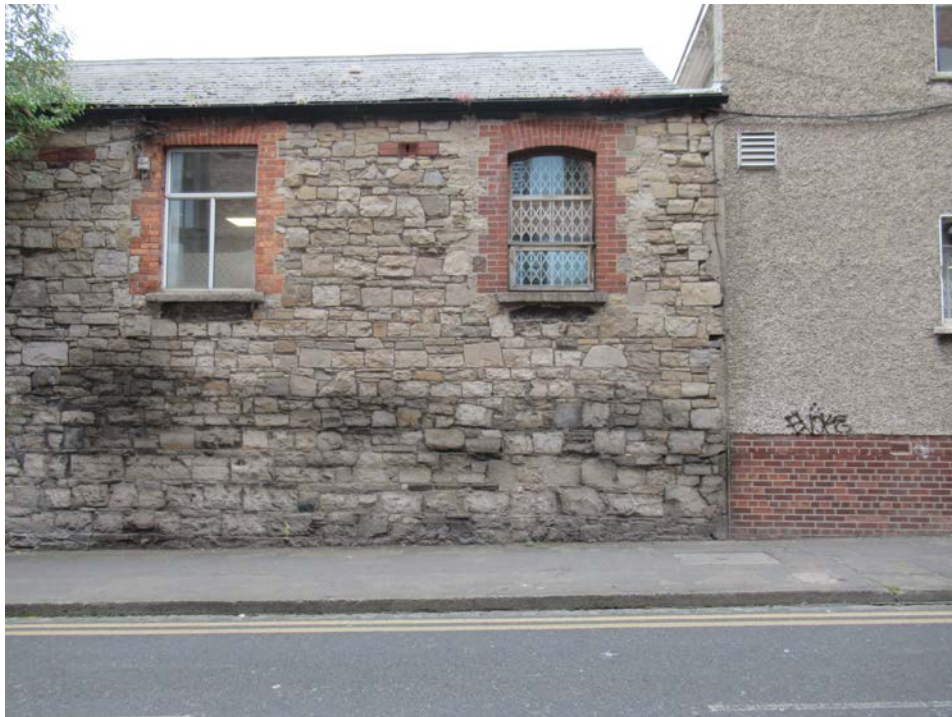
Plate No. 18. Detail view showing the northern end of the east elevation to the L-shaped building, where it abuts the mid-20 th century offices. The L-shaped building originally extended further to the north prior to the middle of the 20 th century. Note the brick surrounds to the windows and simple slated roof.
