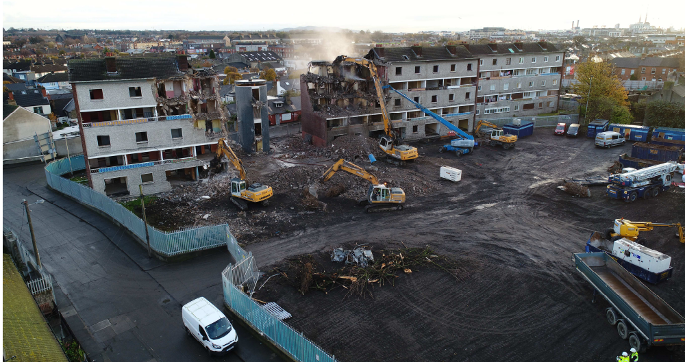
Figures 3A & 3B – Demolition underway at the Croke Villas Site (Tinnelly Group, 2018). Fig 3A ‘Back Block’ removed (foreground) with work underway on two other blocks (No.s 1-21 & No.s 22-42). Fig 3B Aerial view of works with Sackville Avenue to the top of the photo and Ardilaun Square to the left. The Ballybough Railline and Royal Canal run to the bottom of the photo.
