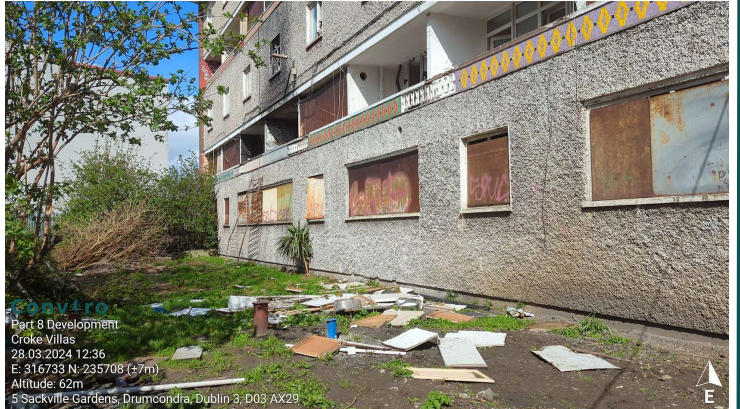
Photo 6: Rear of Croke Villas flats requiring demolition and fly tipped waste visible.
