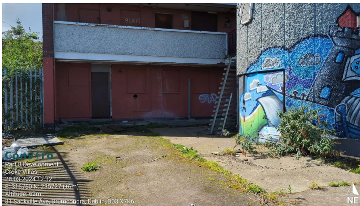
Photo 3: Concrete yard area requiring demolition.
