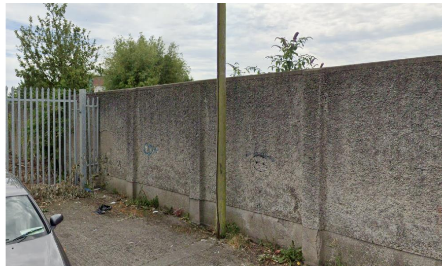
Figure 34: existing boundary wall to railway line removed and replace with stone wall and railings
