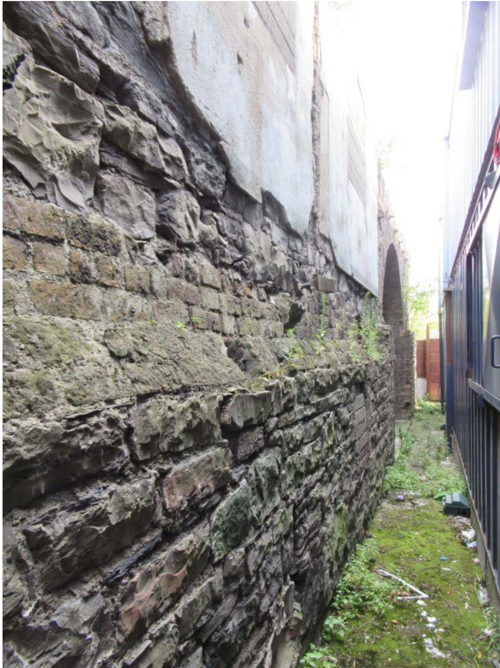
Plate No. 35. General view looking east along the northern boundary to the depot. This view is slightly further to the east than the previous photo, and shows the base of the 19 th century stone and brick masonry wall, formerly an external wall of one of the distillery structures. The arched gate is seen beyond.
