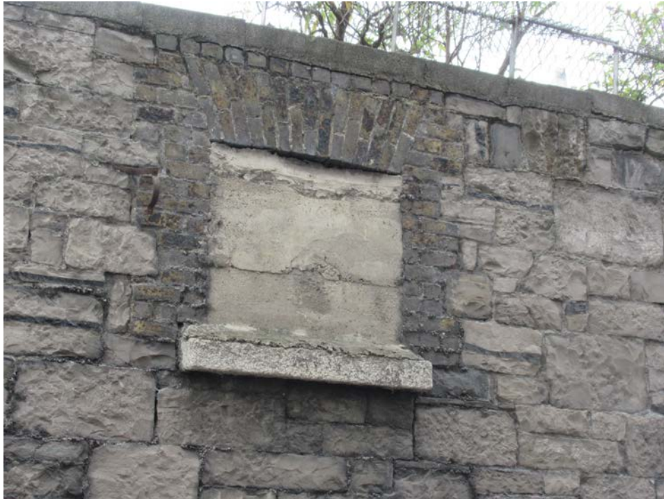
Plate No. 18. General view showing one of the blocked window opening on the Forbes Lane elevation.
