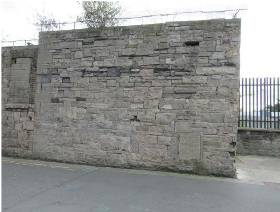
Plate No. 13. General view looking east across the depot, showing the north side of the former Malting House, as well as the remaining corner of the L-shaped structure in the distance.
