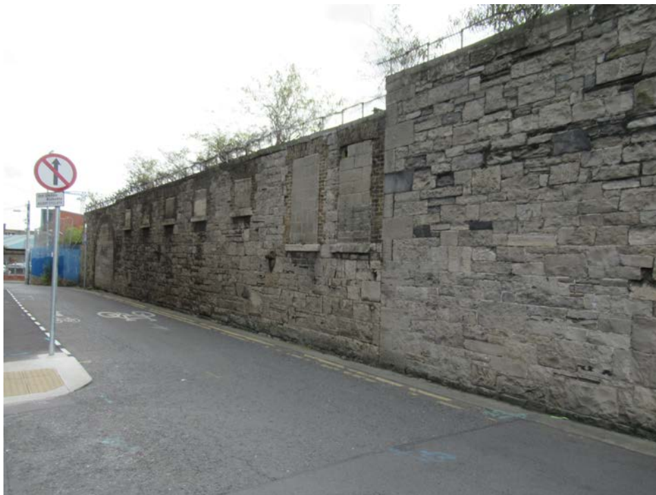
Plate No. 14. General view looking east along Forbes Lane, showing the north side of the former Malting and the other structure with its windows and gate infilled with concrete blocks.
