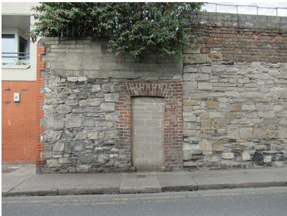
Plate No. 29. General view looking west, showing the southern end of the Marrowbone Lane perimeter wall. This section of wall is comprised of calp limestone rubble with a brick door surround. Of some historical interest, this is a portion of the perimeter wall from the 19 th century distillery.
