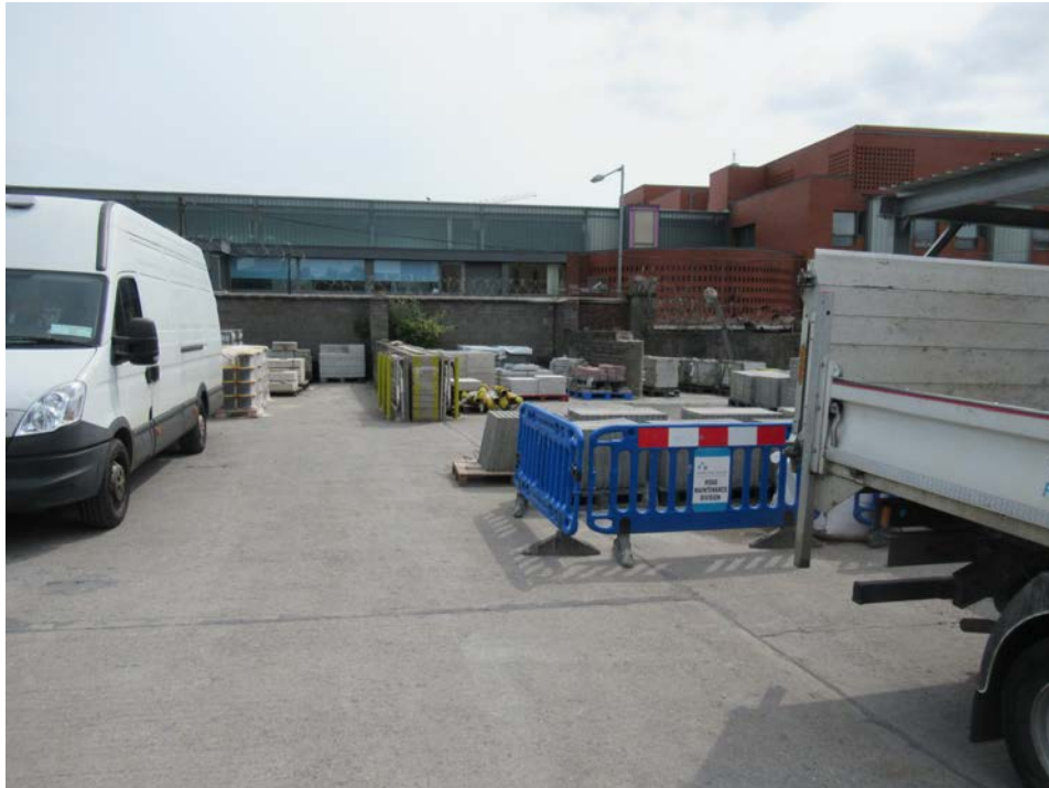
Plate No. 37. General view looking east across the depot, showing the eastern boundary wall. The community centre structure on the east side of Marrowbone Lane is seen behind the wall.
