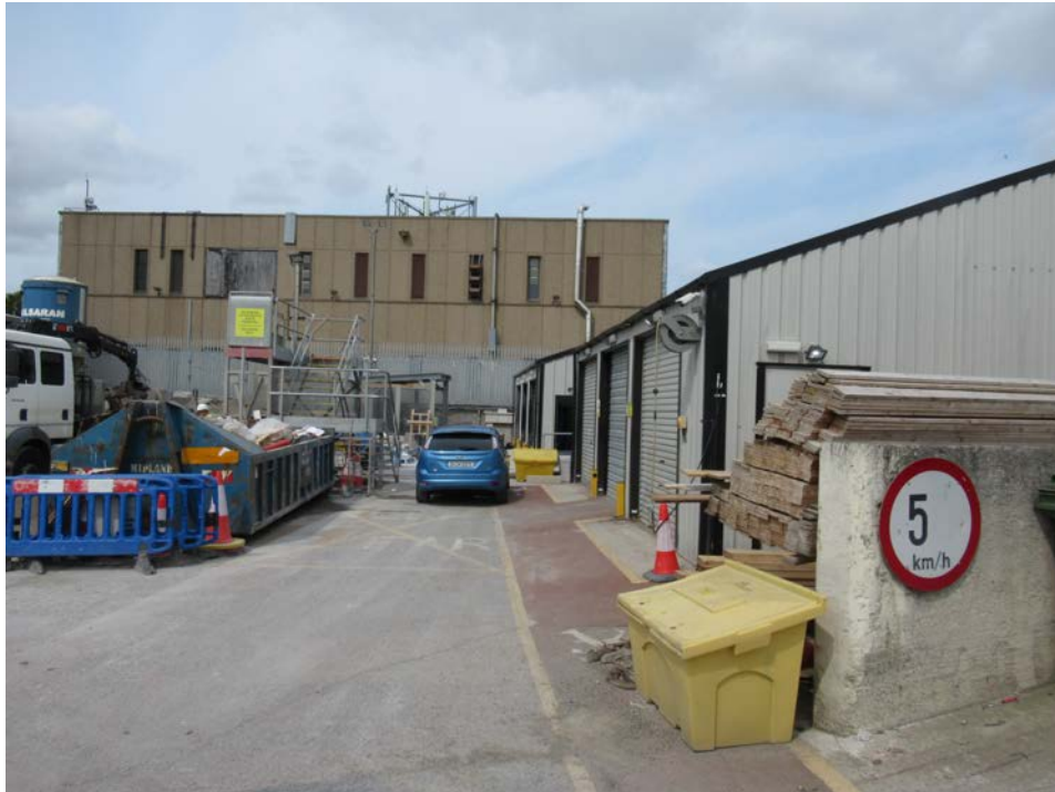
Plate No. 41. General view looking west across the depot site, showing some of the steel framed garages and storage sheds that date from the late 20 th and early 21 st century. The large structure in the distance is the telecommunications complex on the adjacent site.
