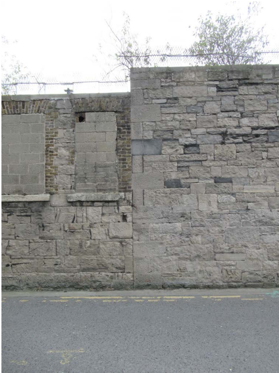
Plate No. 15. General view looking south on Forbes Lane, showing the junction between the two demolished distillery structures. The structure at left was clearly added to the gable end of the large structure to the right. The different types of limestone masonry are evident, along with the brick reveals around the blocked window openings to the left hand structure.
