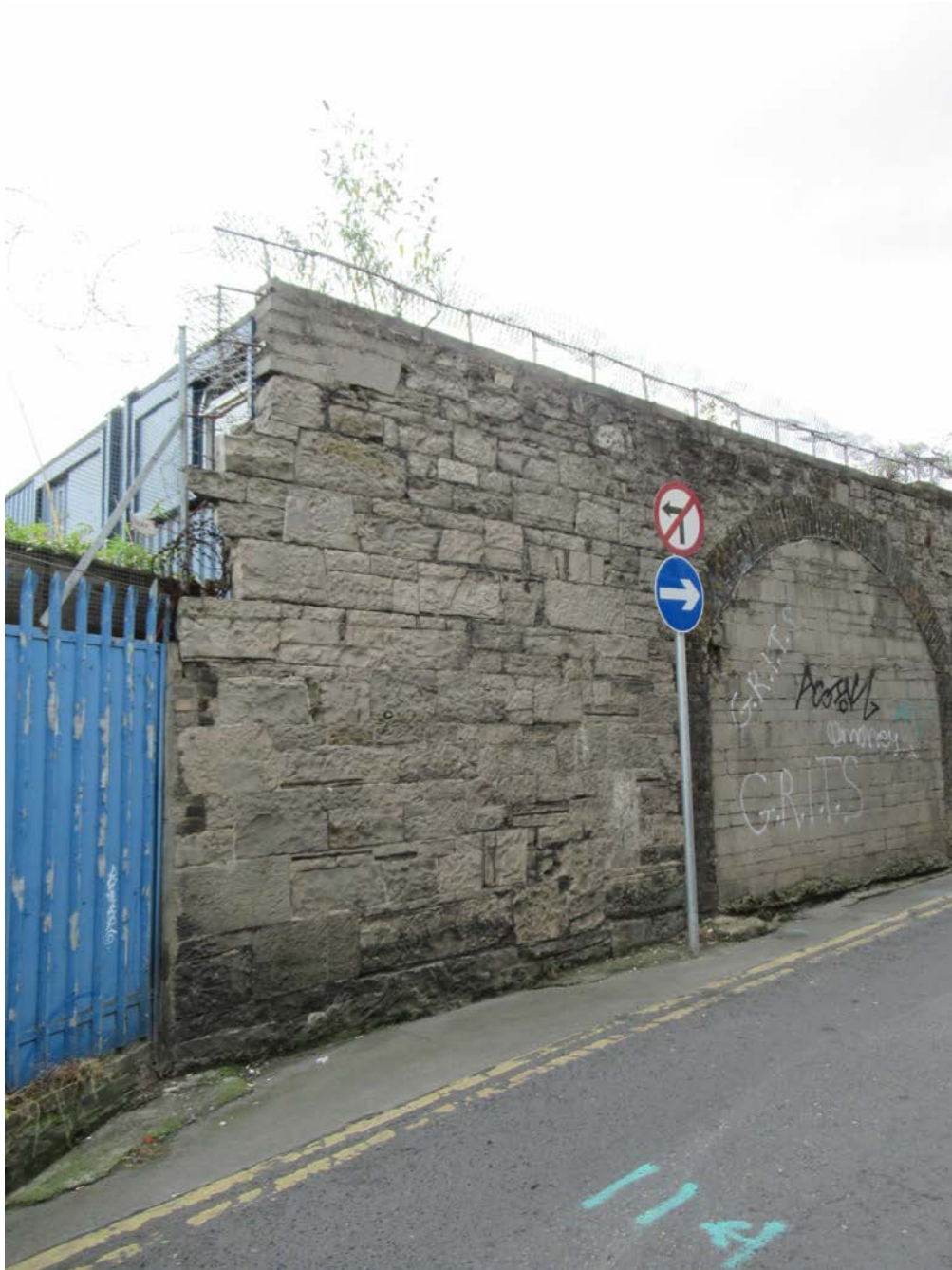
Plate No. 20. General view looking south, showing the east end of the perimeter wall along Forbes Lane. This masonry survives from a 19 th century structure in the distillery and includes a brick arched former entrance gate. The presence of large quoin stones at the left side of the stone masonry shows that the original structure turned the corner at this location. It would make sense to maintain this corner if possible to reduce the cost of cutting back the stone masonry and creating a strong corner.
