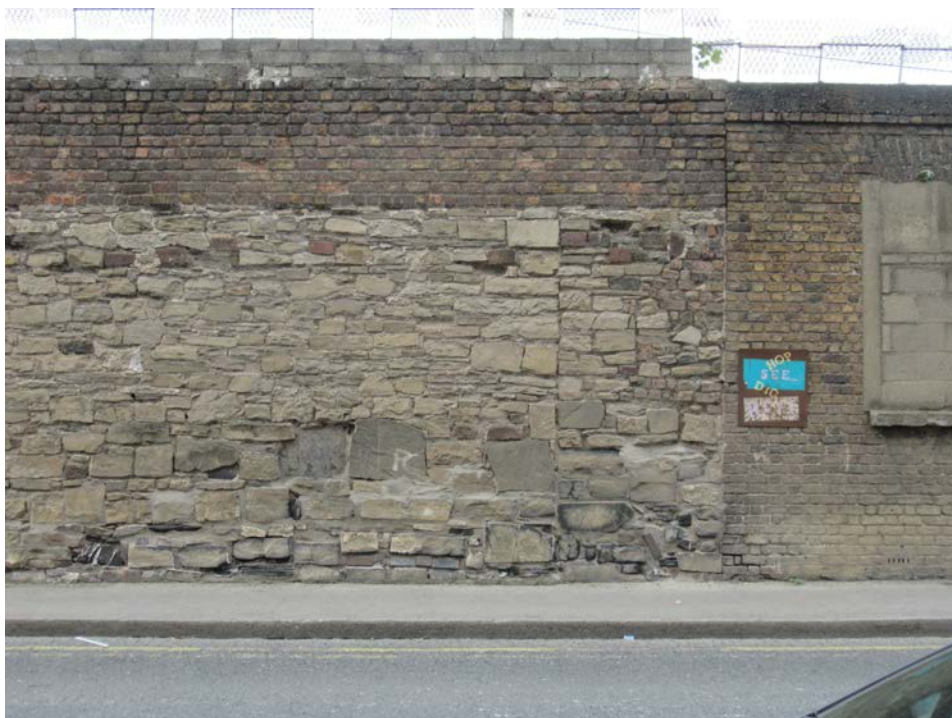
Plate No. 28. General view looking west, showing the rubble stone and brick perimeter wall that stands along Marrowbone Lane, running south from the brick elevation shown in the previous photo.
