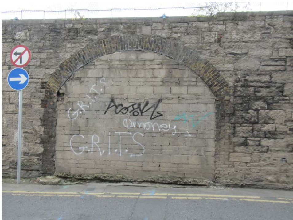
Plate No. 19. General view looking south showing the large arched gate onto Forbes Lane, currently blocked up with concrete blocks.
