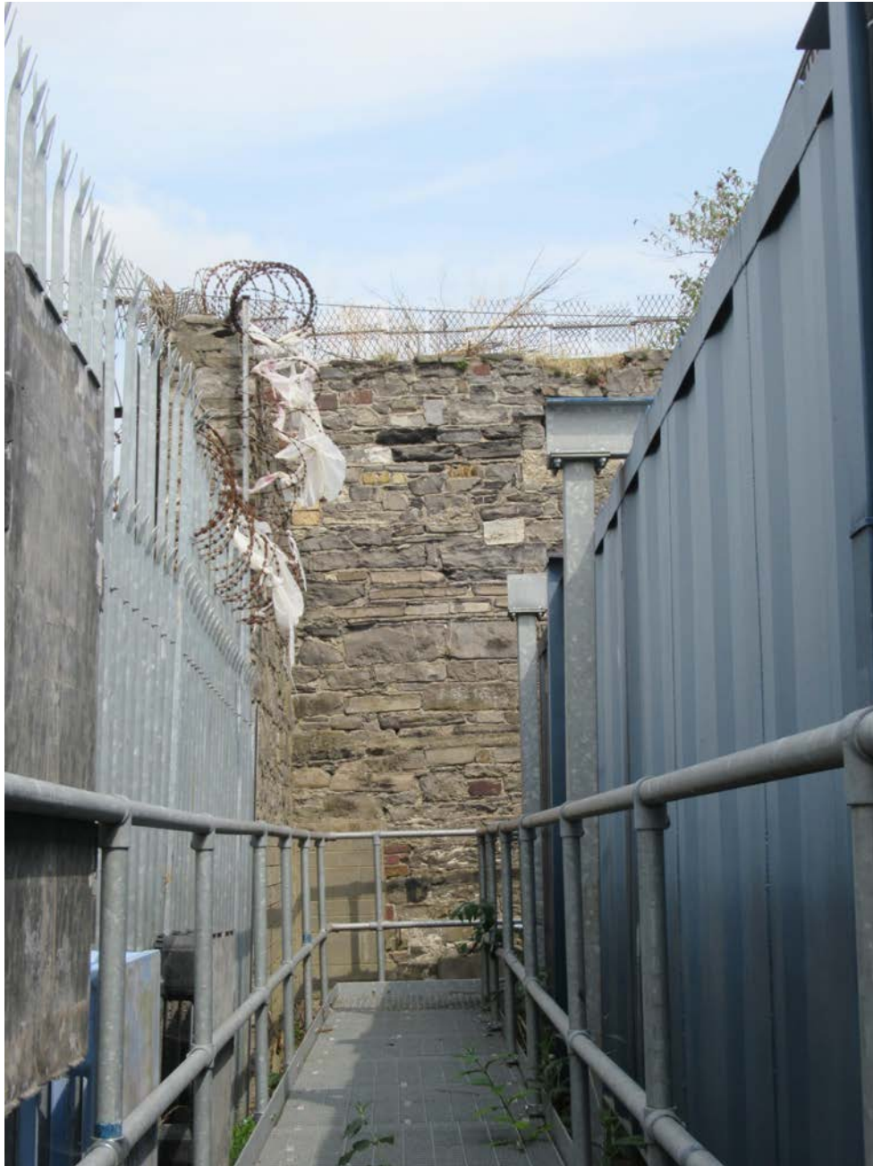
Plate No. 33. General view looking north at the north-west corner of the depot site, showing the inside of the 19 th century stone perimeter wall, surviving from the distillery. This wall is a remnant of one of the large distillery buildings that survived into the middle of the 20 th century, having been adapted for use as a pottery and other uses prior to its eventual demolition.
