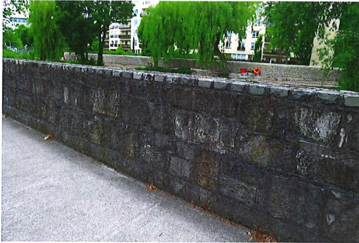
Face of parapet wall from Anglesea Road. Limestone and granite stonework visible with a setts capping.
