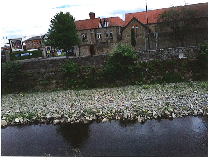
Current view of river wall. Extensive vegetation visible along length of wall.
