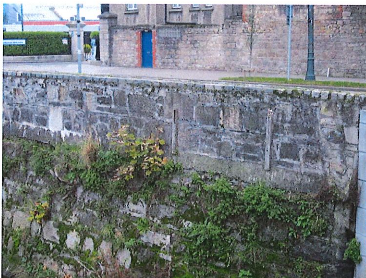
Concrete beam with more recent parapet wall above. Wall capped with sets. Original river wall visible below beam.
