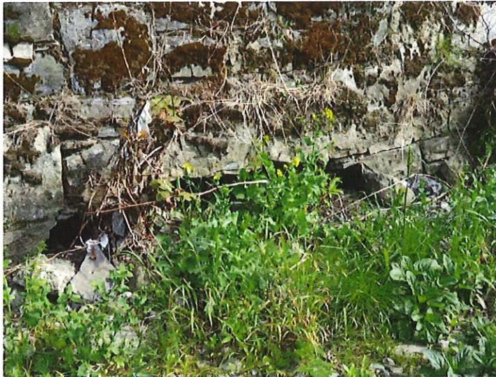
Facing stone lost at low level
