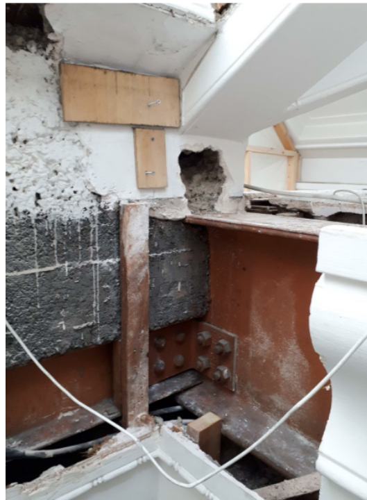
Existing exposed steel to be measured
