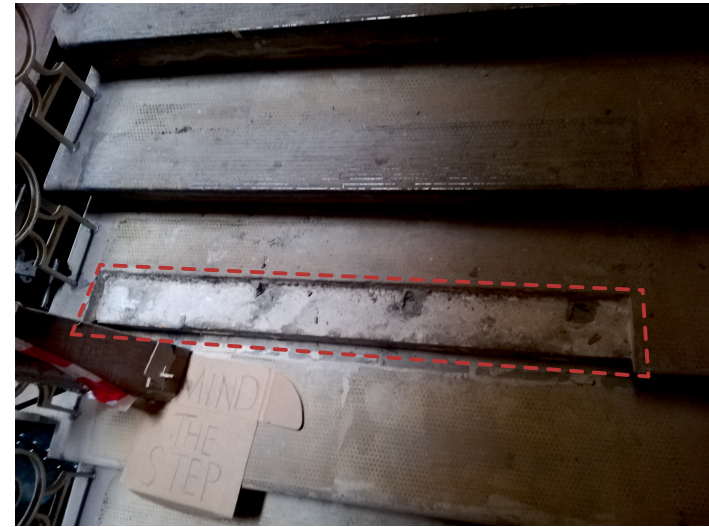
Photograph of the stairs where the metal insert has come loose
