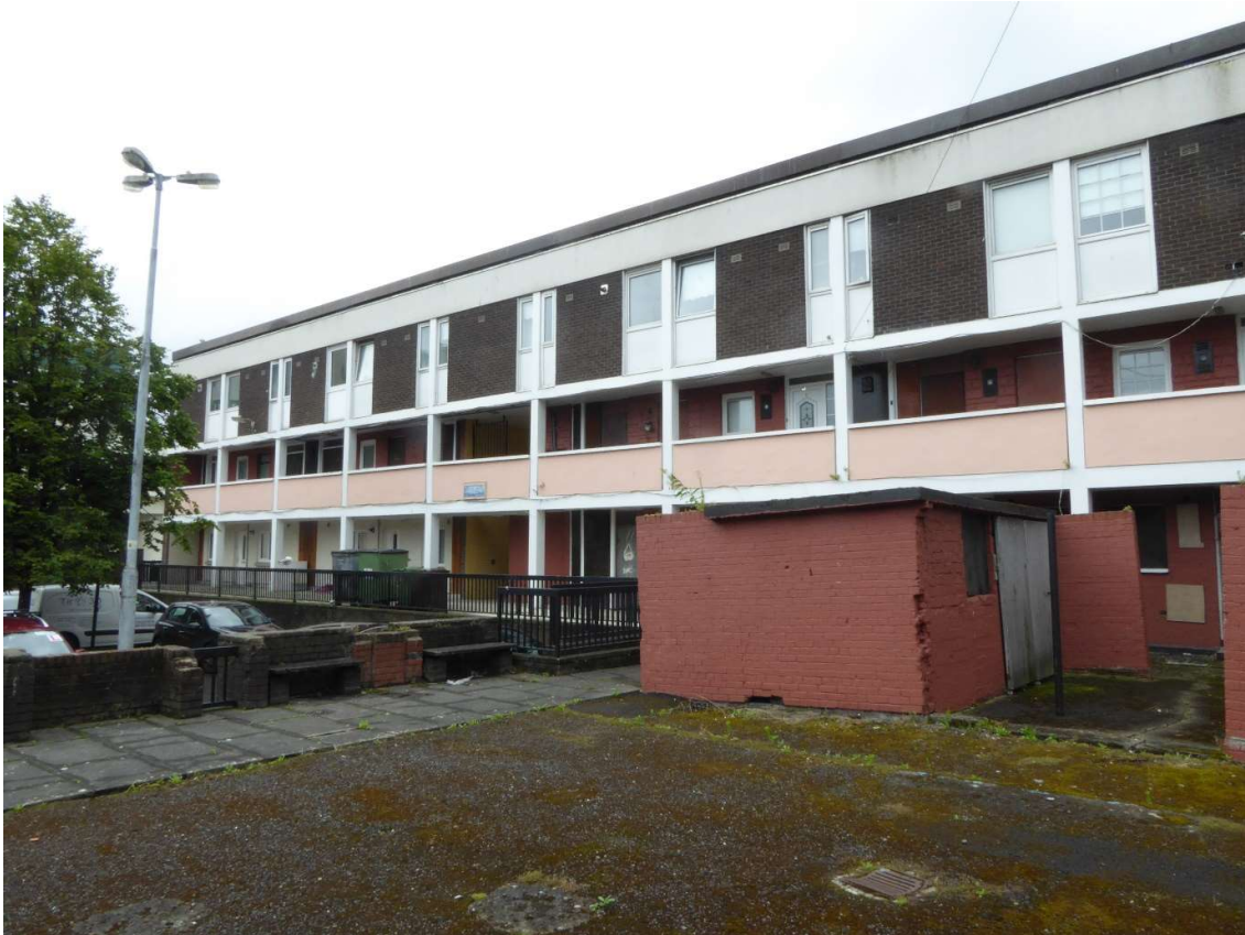
Figure 3 General view of building showing no evidence of birds nesting within the building
