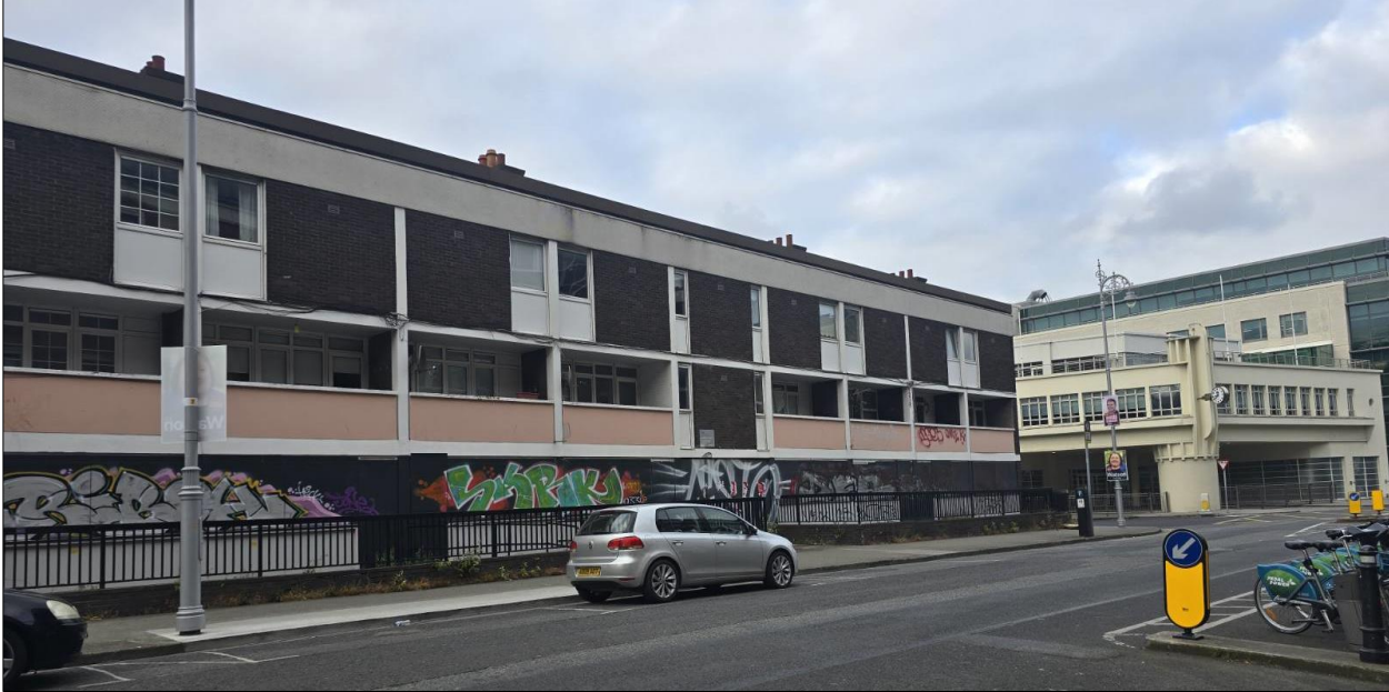
Plate 2 Front of affected structure within city area with Negligible Bat Roost Potential.
