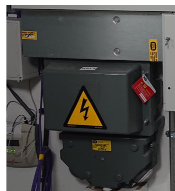
Figure 2: ESB Networks cut-out
