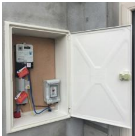
Figure 1: ESB Networks outdoor metering cabinet
