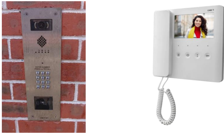
Figure 6: External and internal intercom units
