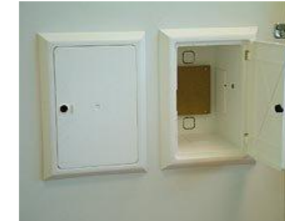
Figure 11: Telecommunications ETU box
