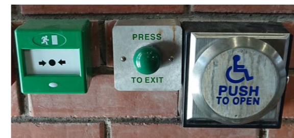
Figure 5: Access control exit buttons
